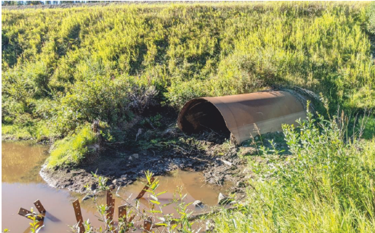
Figure 2-3: Main Culvert Crossing debris blockage at inlet in August 2022
