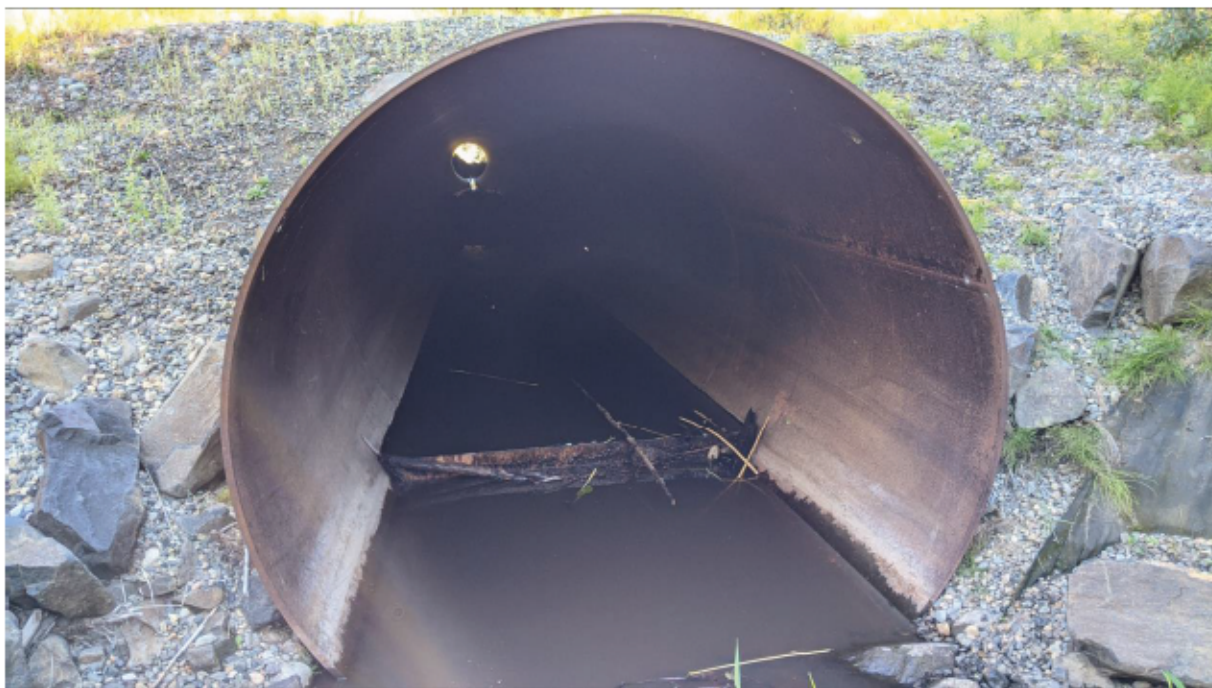
Figure 2-4: Main Culvert Crossing facing upstream from the outlet; note the lack of embedment (August 2022)
