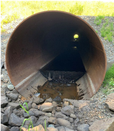
Photo 5: View upstream of the 2400 mm steel culvert and baffles where fish were observed.
