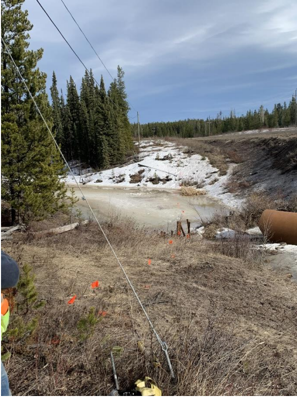
Photo 33 Marked Utility line From Western Pole near STA 105+00
