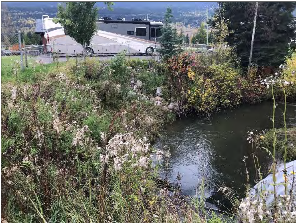
Figure 18: Erosion of the south bank approximately 8 m upstream of the culvert inlet
