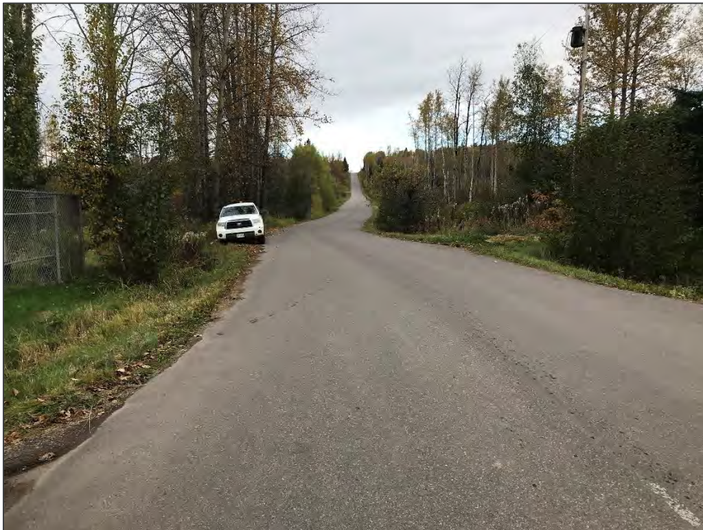
Figure 23: View north on Henry Road from south of the existing culvert on Kathlyn Creek.
