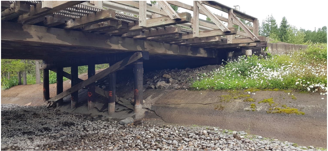
Photo 3: Spawning channel left bank, looking upstream. Note crack in concrete at piles (August 15, 2020).
