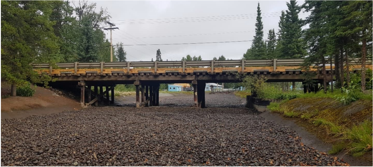
Photo 1: Fulton Bridge crossing Spawning Channel, looking downstream towards fish fence. Note concrete banks and gravel channel bottom (August 15, 2020).
