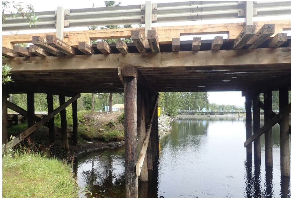
Photo 7: Fulton River crossing, left bank, looking downstream. Note eroded outside corner with no riprap at bridge, and riprap berm downstream of bridge (August 15, 2020).
