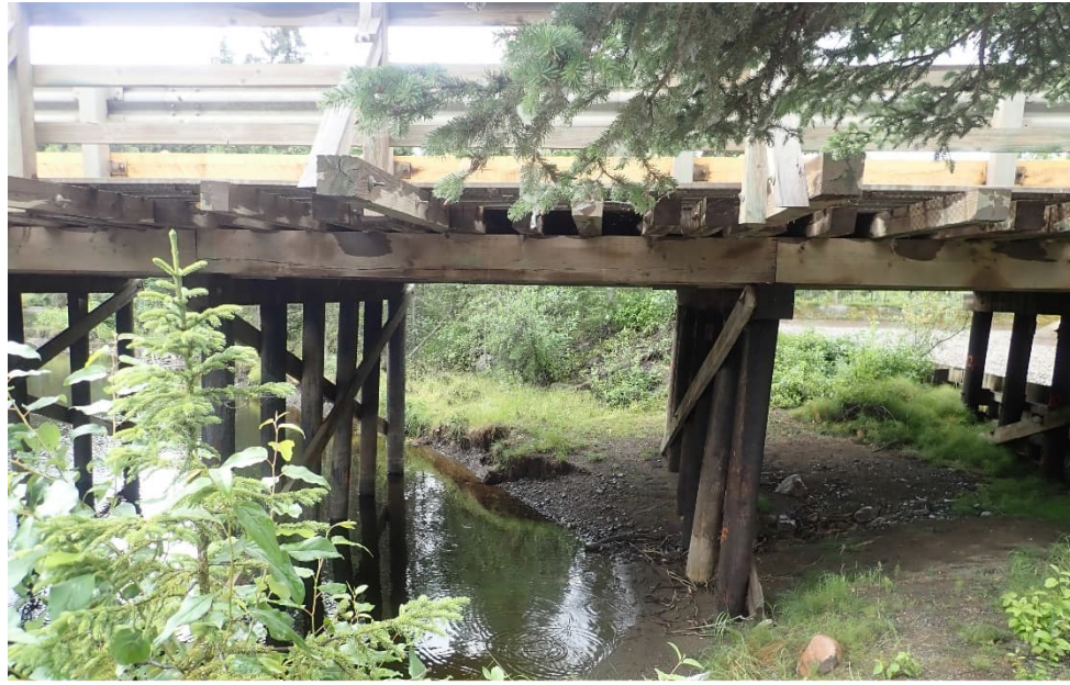
Photo 5: Fulton River crossing, left bank, looking upstream. The left bank is the outside corner after a sharp bend. Note the erosion, and low elevation of the bank relative to the wood wall for the spawning channel (August 15, 2020).
