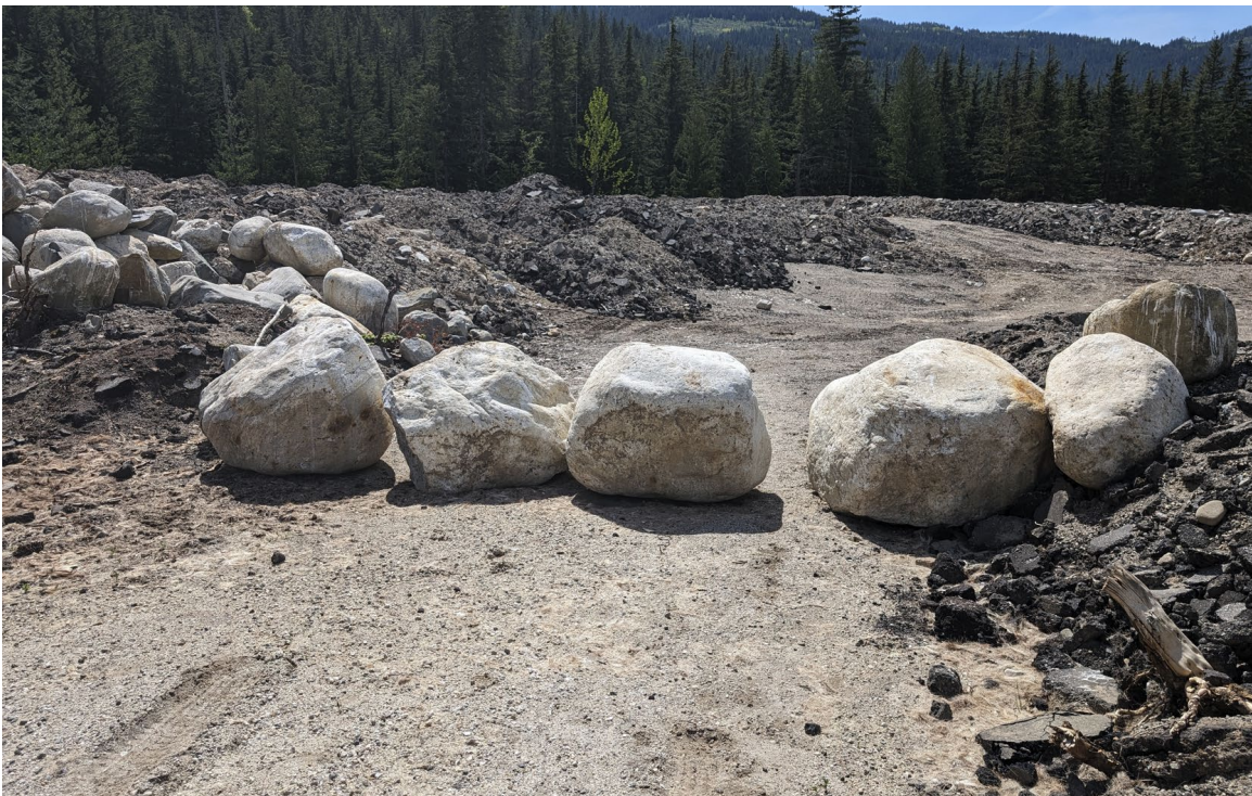
Access into newly developed area near asphalt piles is blocked by boulders (May 2024).
