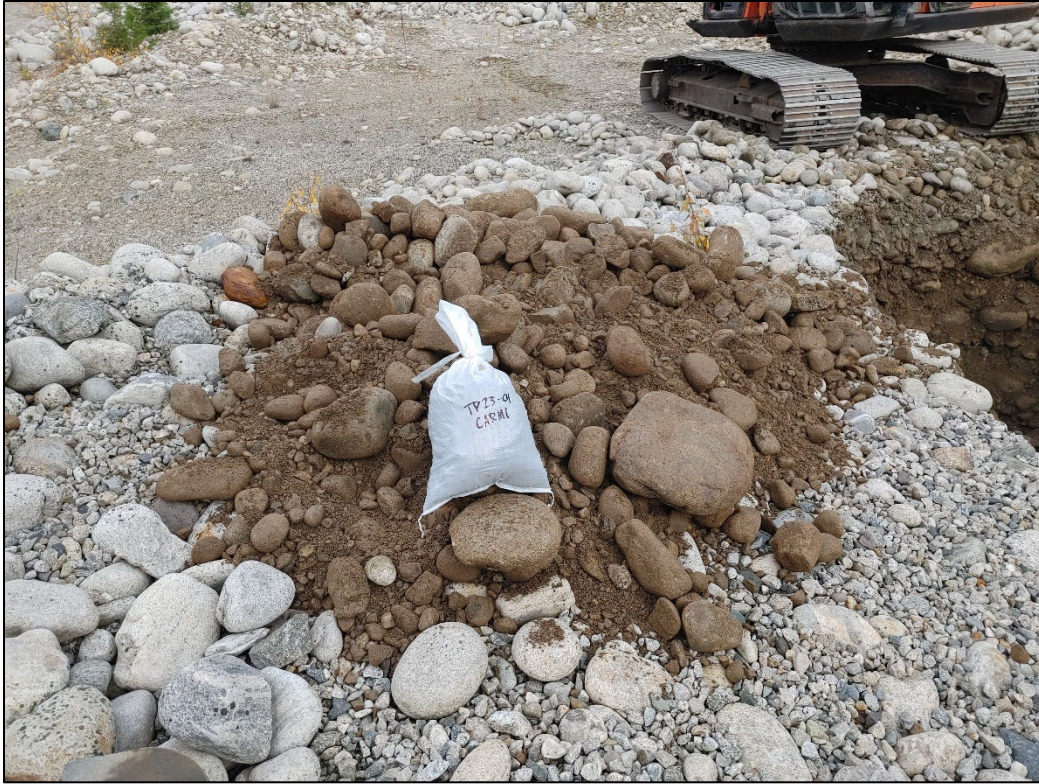
Photo 3 TP23-01 spoil pile. Note the amount and size of large boulders (October 2023).
