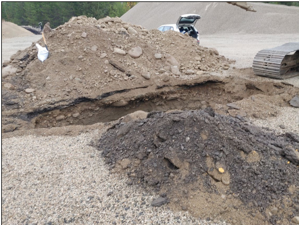
Photo 8 TP23-11 in the northern portion of the pit. Note the asphalt layer at the surface (October 2023).
