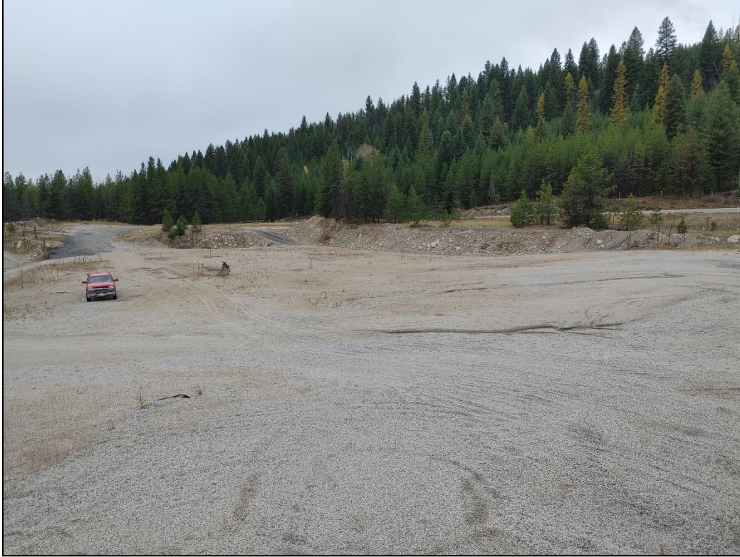
Photo 1 Crusher set-up area and stockpile space to the right closer to highway; mining area on the left (October 2023).
