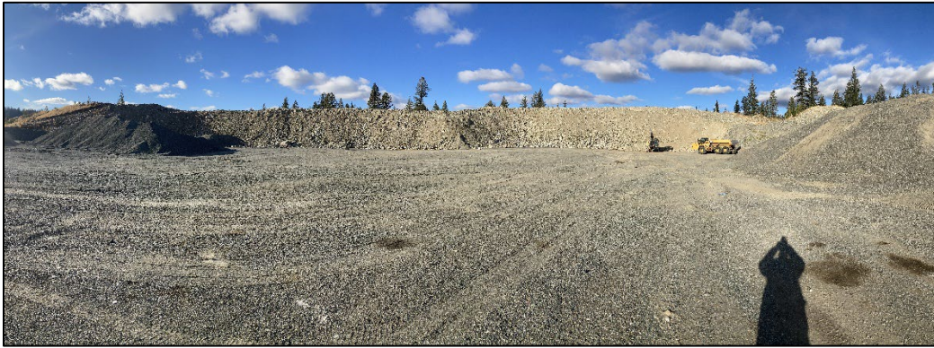
Photo 3 View: northwest. Pit face with proposed crusher and stockpile location in the foreground. Note: mining has taken place since the photo was taken (November 2022).
