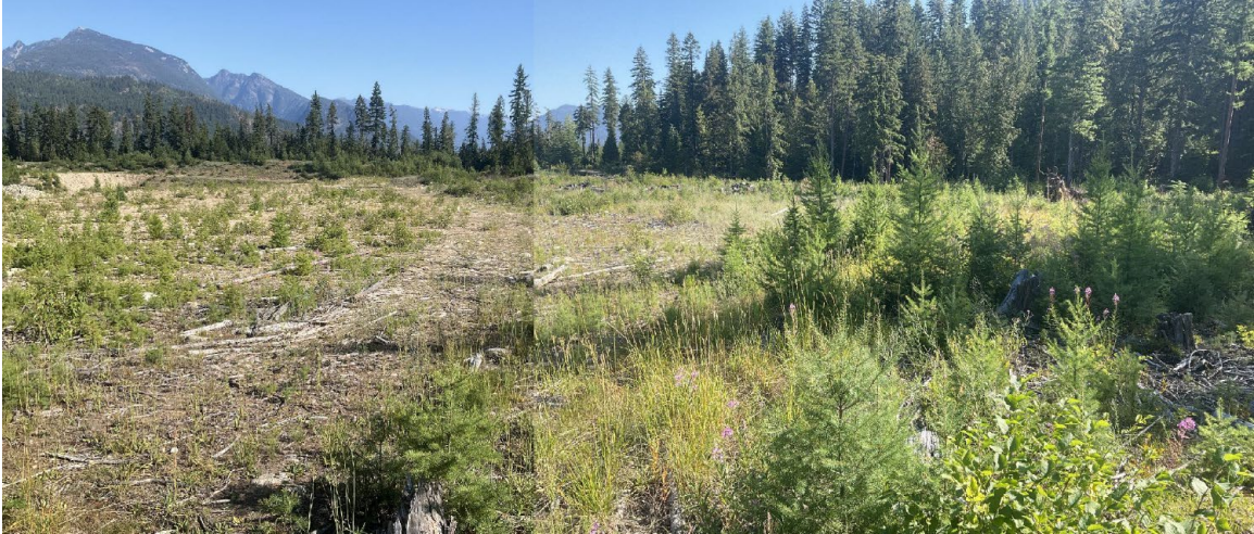
Cleared and partially grubbed/stripped in eastern portion of Area A (near TP93-12)
