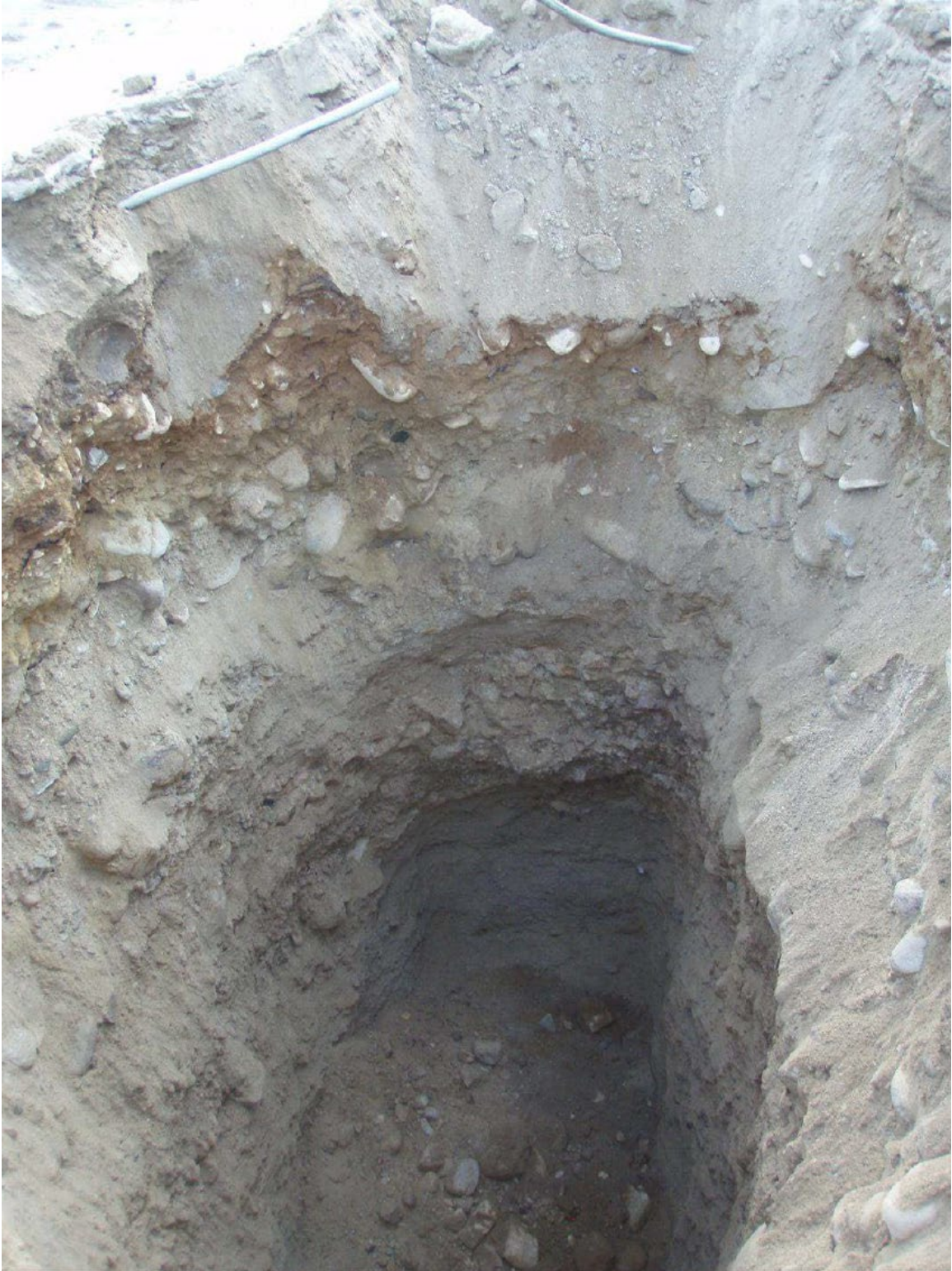
TP14-18 - note material near top of hole may be buried posts or other construction waste material
