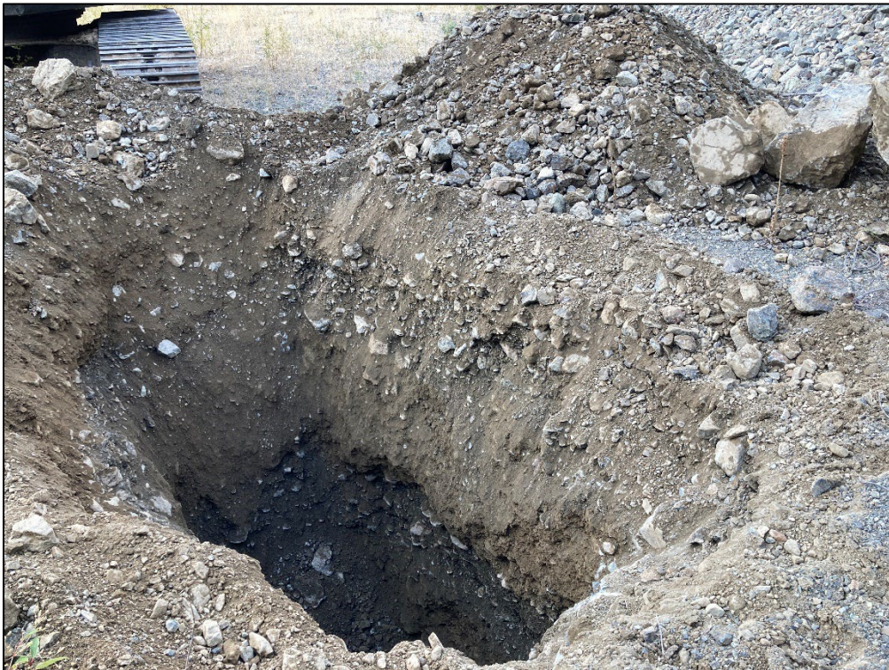
Photo 6 TP21-10 test pit and spoil pile (well-graded gravel). Test pit is located on the pit floor at the base of the pit face (Oct. 2021).
