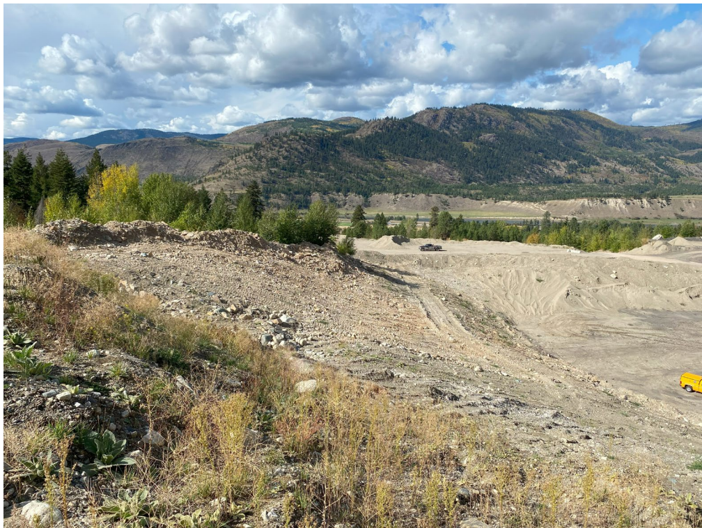
West view into leased area of pit with potential stockpile location in background where truck is parked, September 2023.
