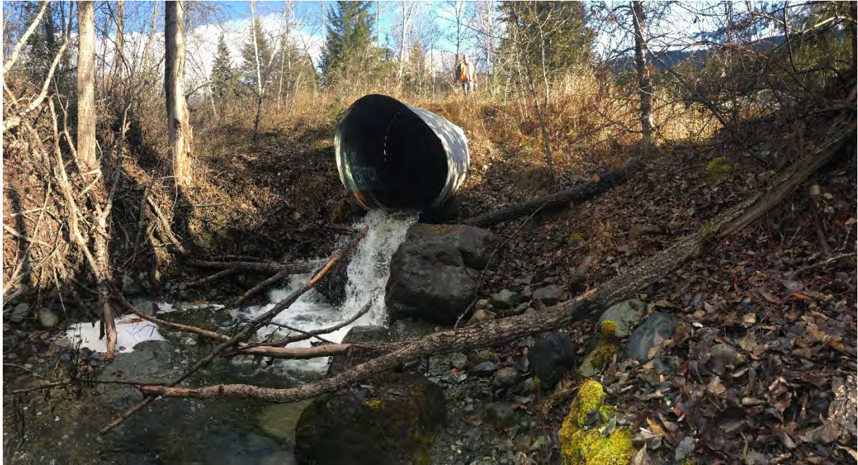
Figure 2-5. Upstream view of Newhykulston Creek culvert outlet at Dunn Lake Road. Note the approximate 1 m drop. BGC photograph of November 28, 2018.
