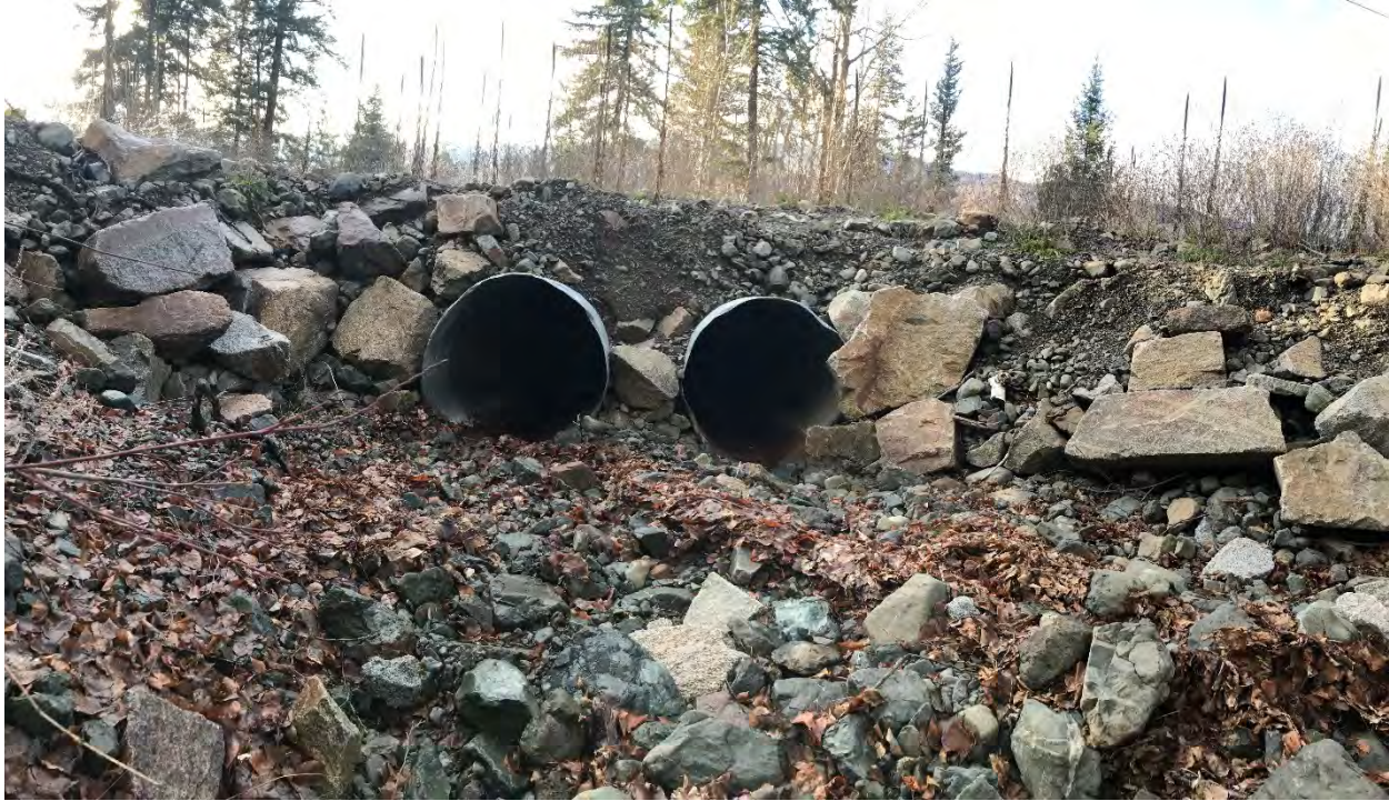
Figure 2-9. Downstream view of Skowootum Creek twin 1.2 m CSP culvert inlets at Dunn Lake Road. BGC photograph of November 28, 2018.
