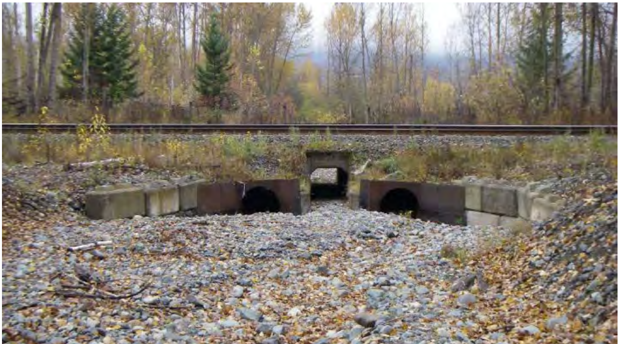
Figure 2-6. Downstream view of Newhykulston Creek at the CN Rail crossing (from M.J. Milne & Associates Ltd., 2012). Channel aggradation appears to be occurring upstream of the crossing.
