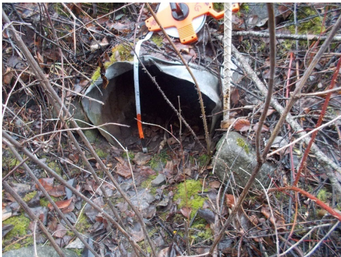
Photo 23. Watercourse-ID 4 - 500mm CSP at inlet, no sign of recent flows
