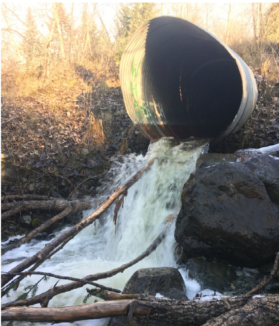
Photo 7. Newhykulston creek - 1800mm CSP creating fish barrier to upstream fish migration
