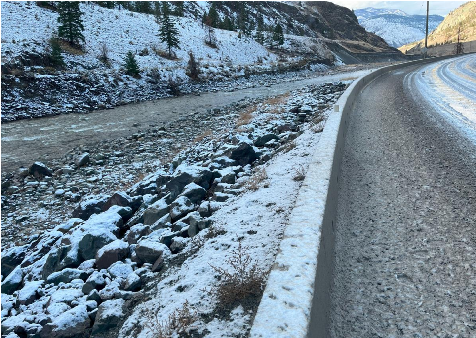
Photo: Site 16/17 transition illustrating riprap voids.
