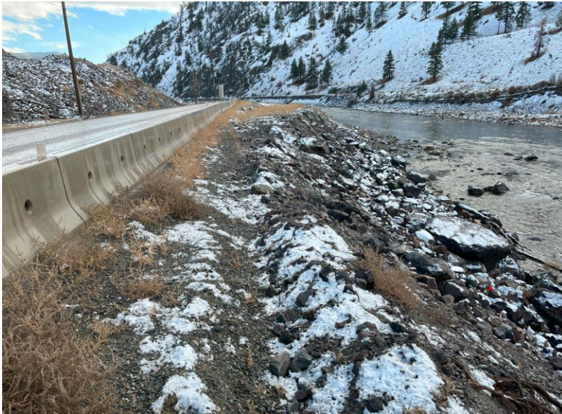
Photo: Site 17 photo of northwest end, view upstream close to transition back to existing pavement
