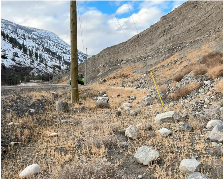
Photo: Site 18 view north of the north end illustrating existing steep slopes from event and silty sand material in ditch.
