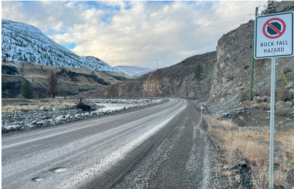
Photo: Site 19 view to north illustrating riprap, slopes and localized road surface feature.
