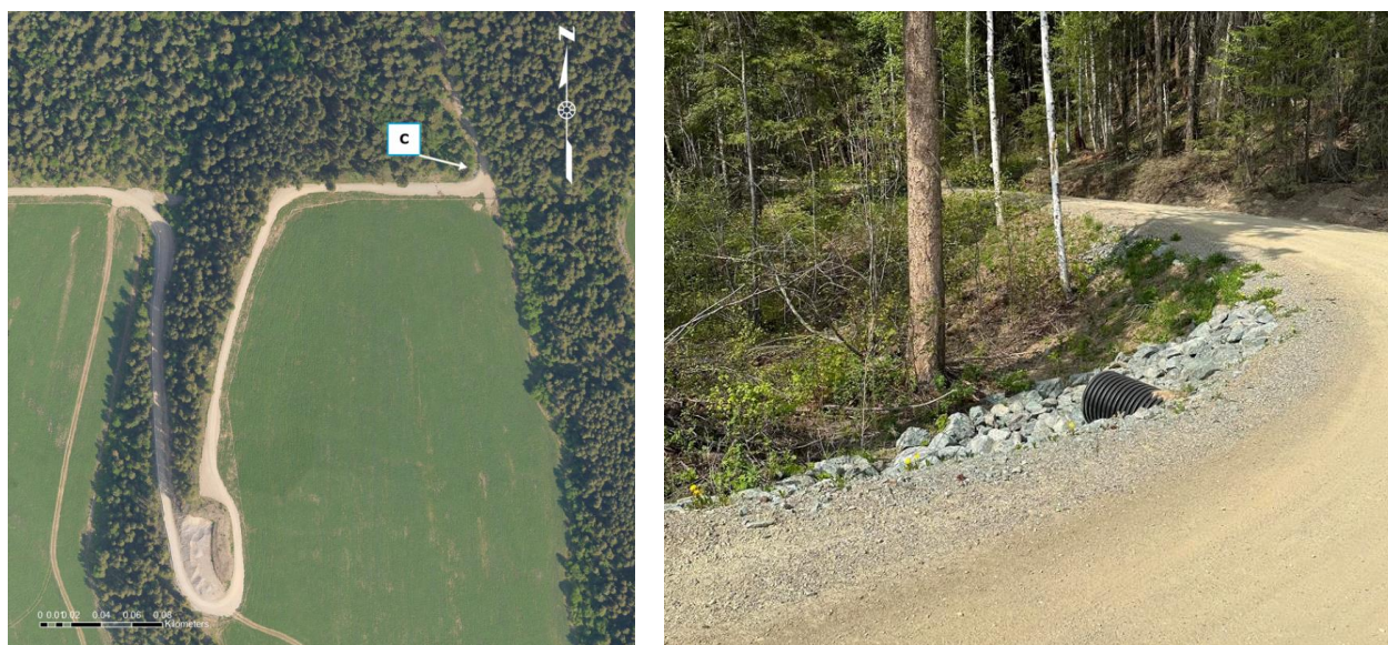
Figure 4 – Location ‘C’ crossing of an unnamed drainage course was dry during the inspection. Left image: Site location. Right image: Site photo during the inspection
