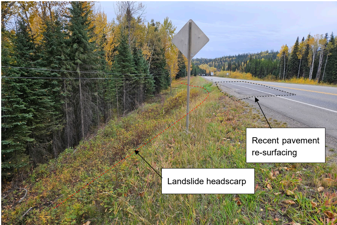
Photo 1 Landslide headscarp encroachment on highway, looking north, Sept. 25, 2023.
