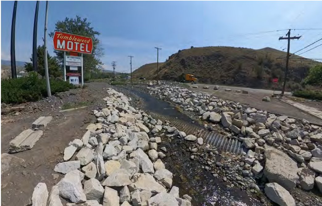
Reach 2 Site 1 destroyed former Quartz Rd facing upstream.
