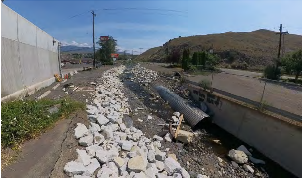
Reach 2 damaged former Quartz Rd culvert and emergency riprap.
