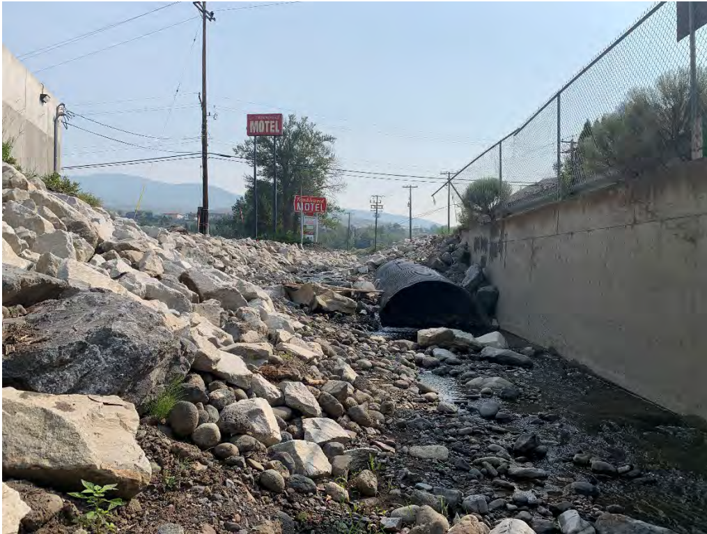
Reach 2 Site 1 washed out Quartz Rd culvert and emergency riprap.
