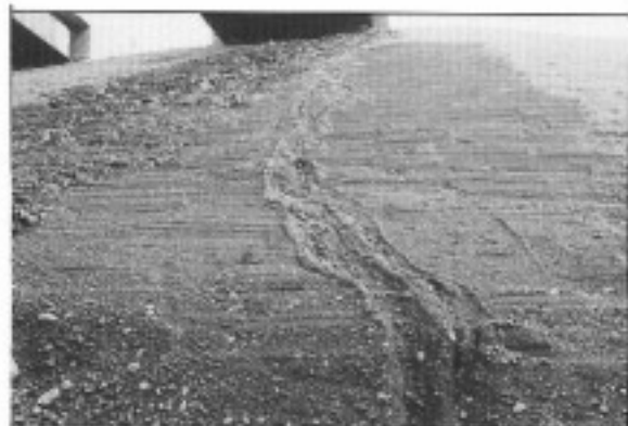
Fig. 21 Erosion from deck drainage.
