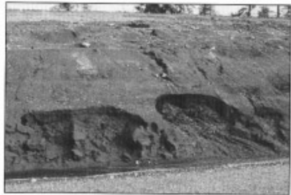
Fig. 12. Failure in a sand stratum with a high water table
