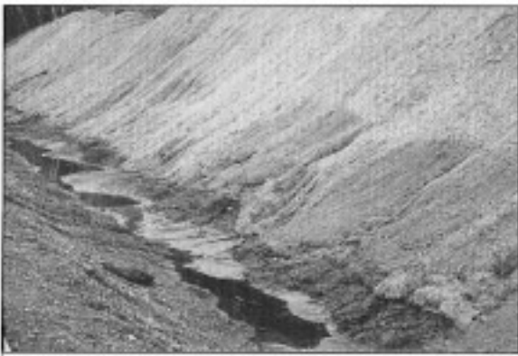
Fig. 20 Erosion under a manufactured blanket.
