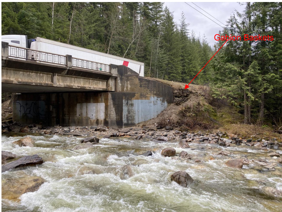
Photograph 4. View looking east (upstream) at the downstream wing wall of the east abutment. (Photograph by BGC taken on April 26, 2023).
