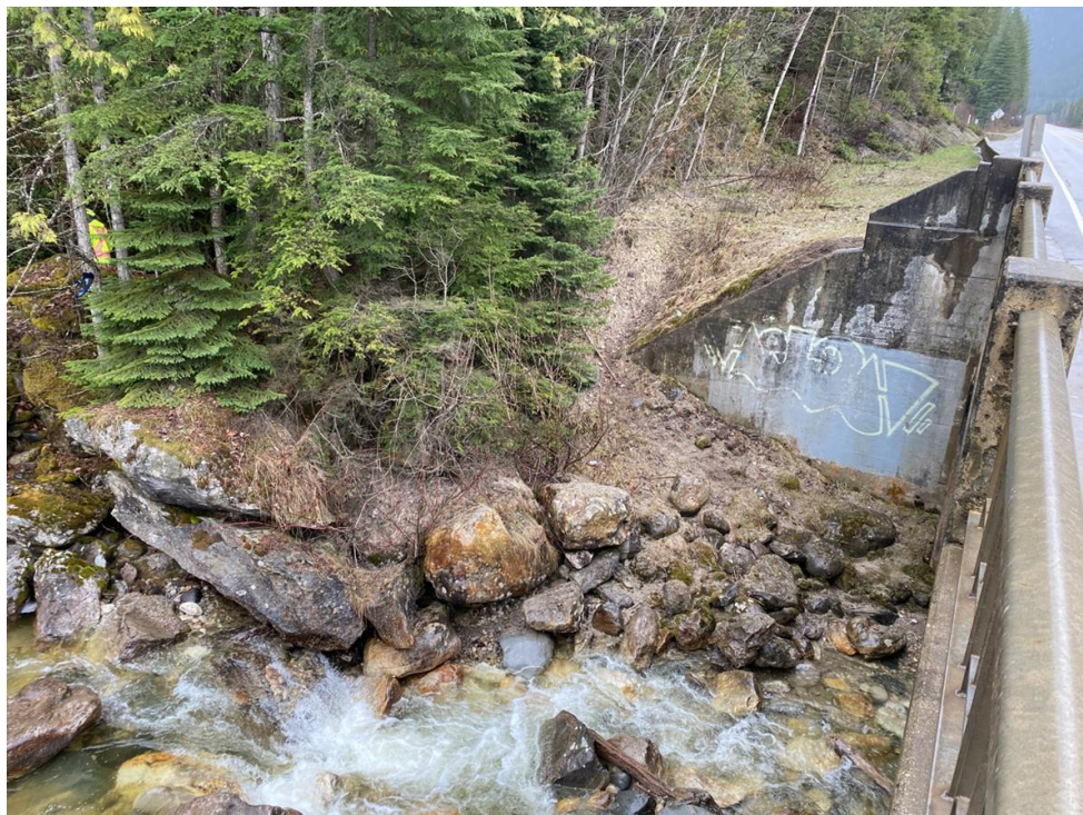
Photograph 2. View looking east at the upstream wingwall of the east abutment (Photograph by BGC taken on April 26, 2023).
