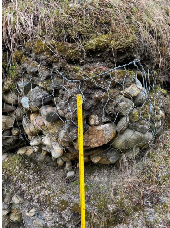
Photograph 11. View looking northwest damaged/disconnected wiring on the gabion basket (Photograph by BGC taken on April 26, 2023).
