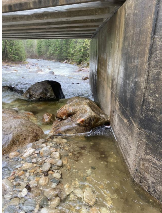
Photograph 7. View looking south (downstream) at the west abutment foundation wall (Photograph by BGC taken on April 26, 2023).
