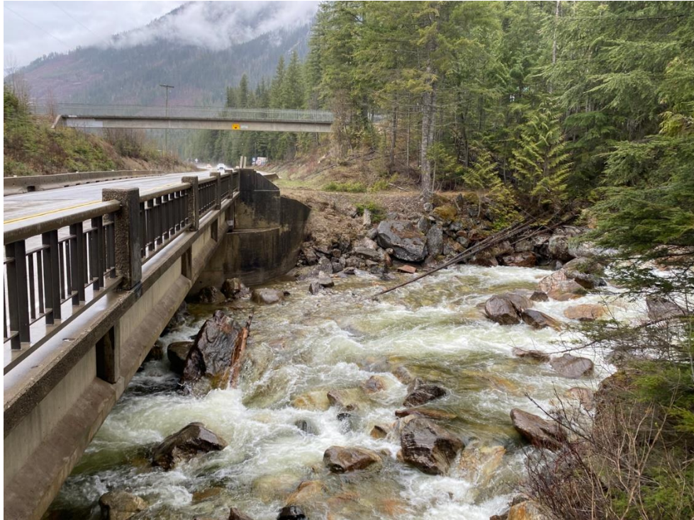
Photograph 9. View looking northwest at the upstream wing wall of the west abutment (Photograph by BGC taken on April 26, 2023).
