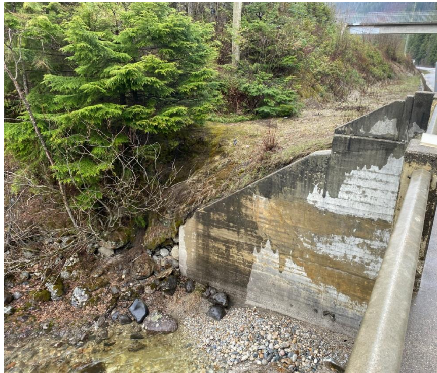
Photograph 5. View looking west at the downstream wing wall of the west abutment (Photograph by BGC taken on April 26, 2023).
