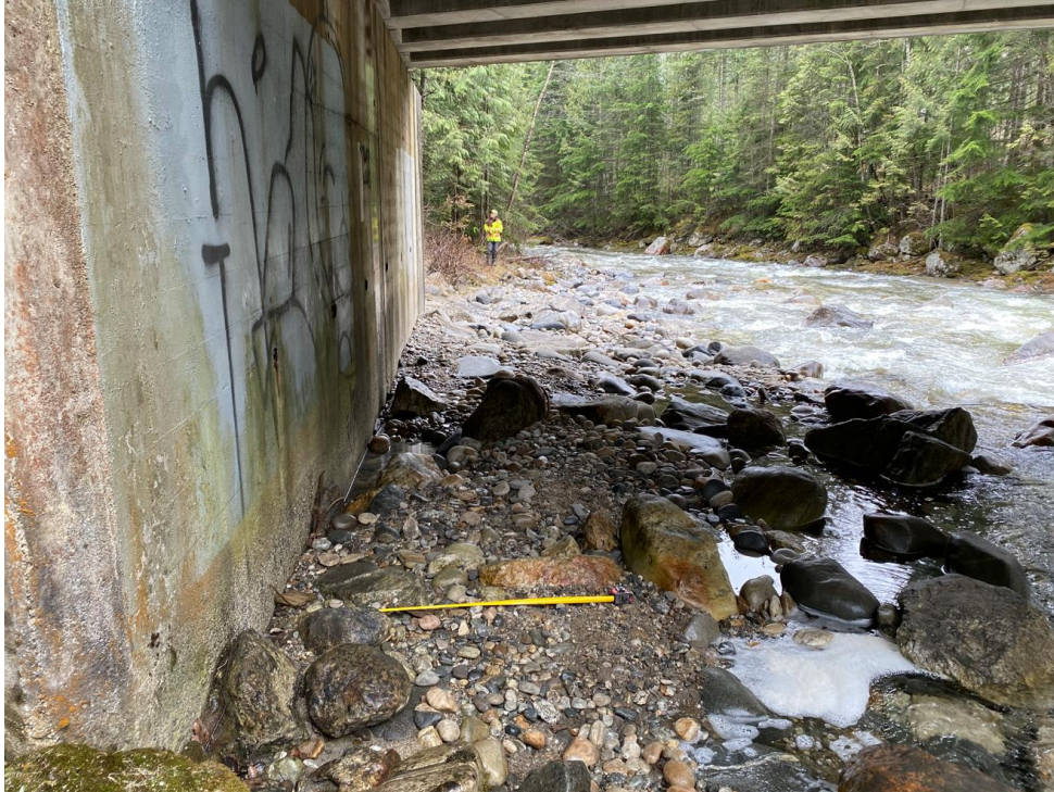
Photograph 3. View looking south (downstream) along the east abutment foundation wall. The measuring tape is extended to 1 m in the photo (Photograph by BGC taken on April 26, 2023).
