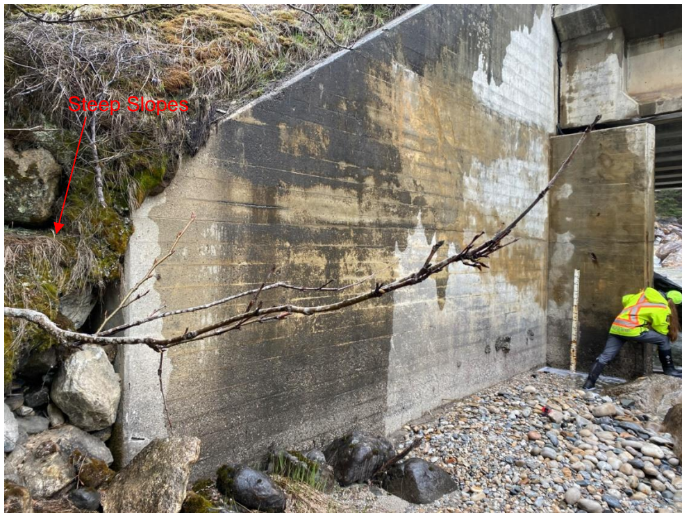
Photograph 6. View looking north (upstream) at the downstream wing wall of the west abutment (Photograph by BGC taken on April 26, 2023).
