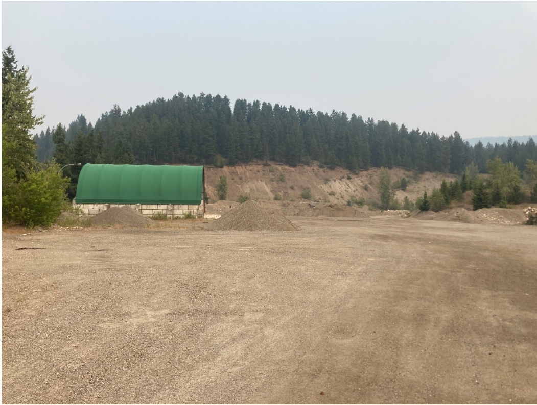
Crusher set up in background right of the salt shed, stockpile space at left. July 2021.
