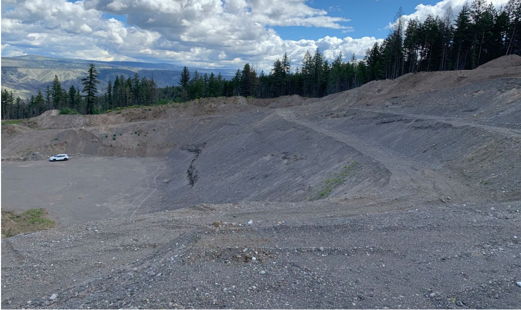
Figure 3 View of pit face, looking east. The dirtier material visible in the top right corner of this photo is the overburden requiring relocation (July 2022).
