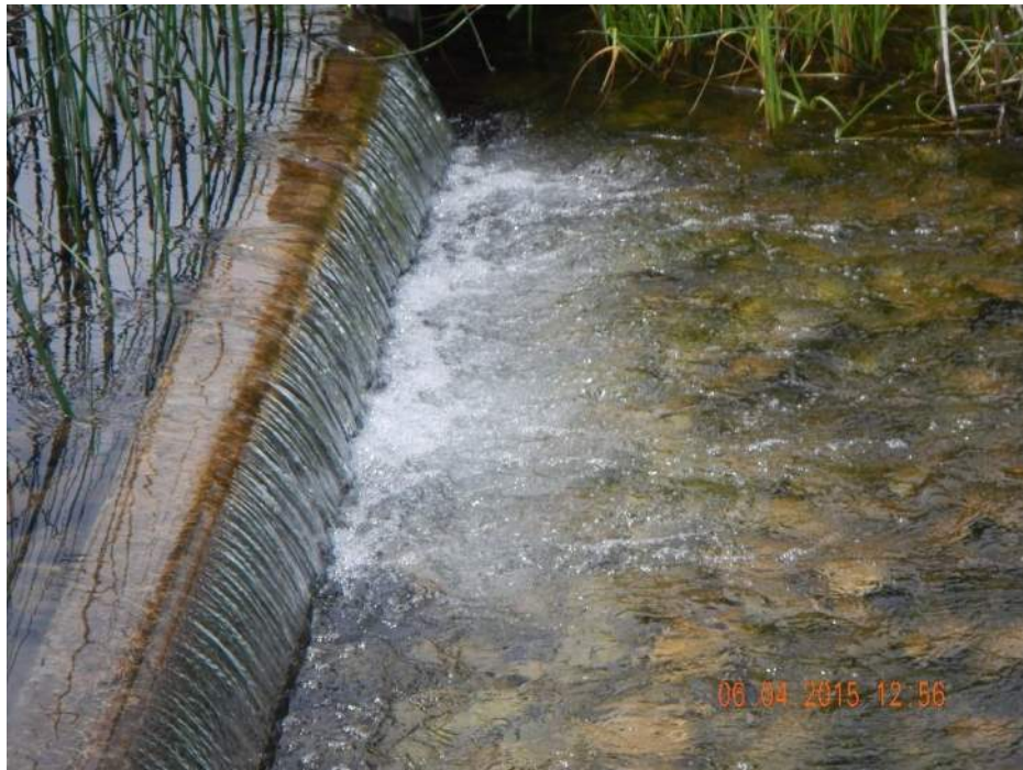
Figure 3-4: White Lake Outlet Control Structure
