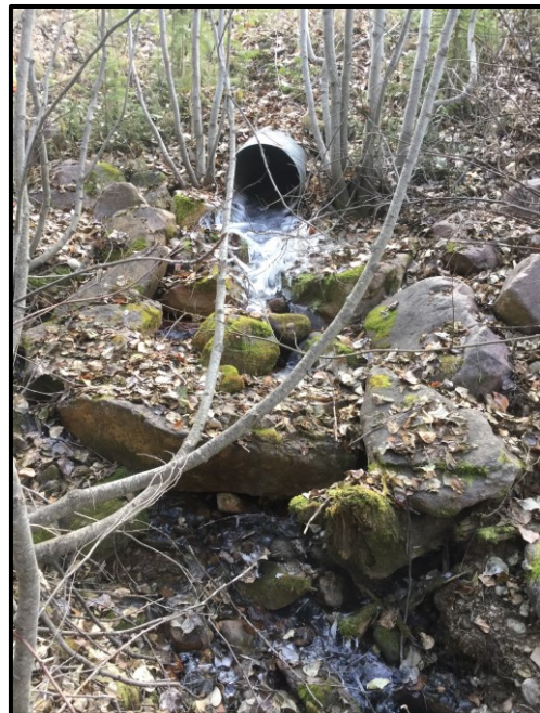
Photo 8: Large boulders at the outlet of culvert C131, Stream 13.
