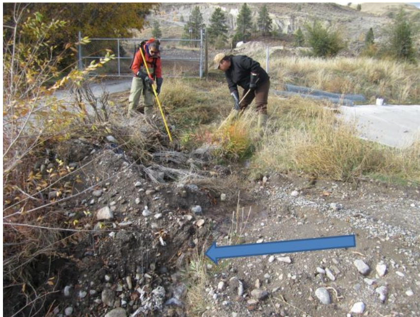
Photo 4-2: Construction alteration of Skaha Creek above Highway 97 at Site 2. Slumping, erosion, and sediment transport has occurred, indicated by the blue arrow.
