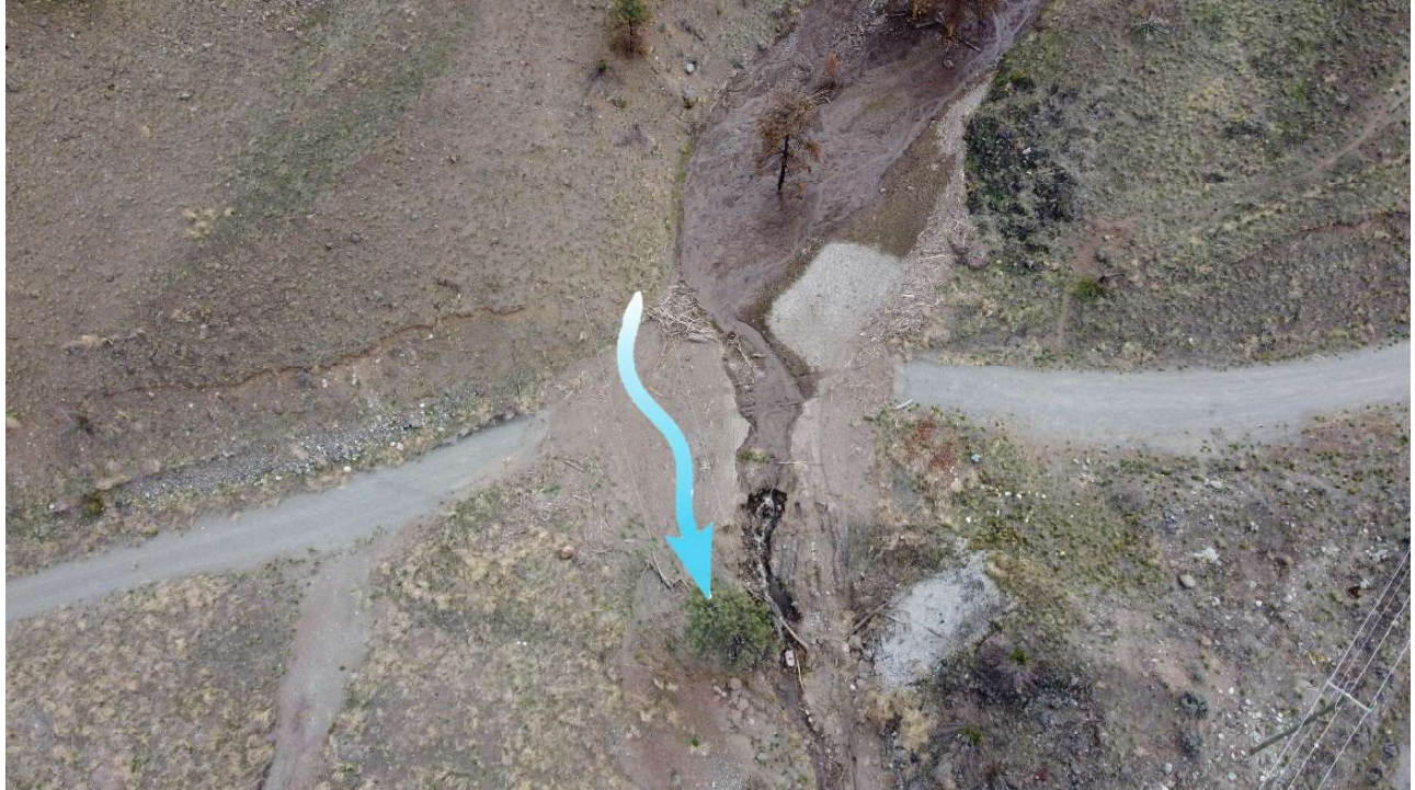
Figure 2.5 Sackum Creek eroding through access road, blue arrow denotes flow direction
