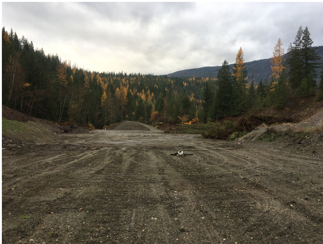
West view of crusher set up in foreground, overburden stockpile to left. October 2018.
