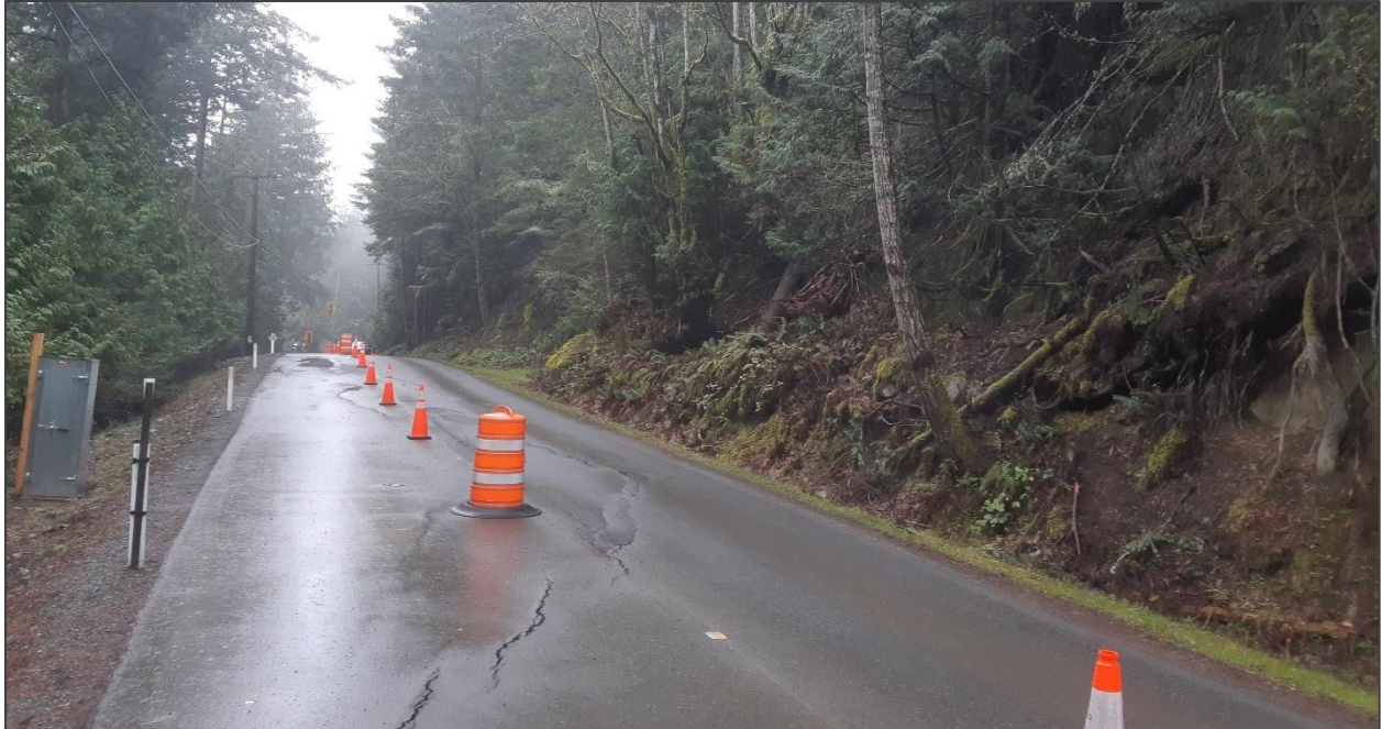
Figure 2. Canal Road on South Pender Island, BC - image of the longitudinal pavement crack and steep terrain above the road (view from the West to the East).
