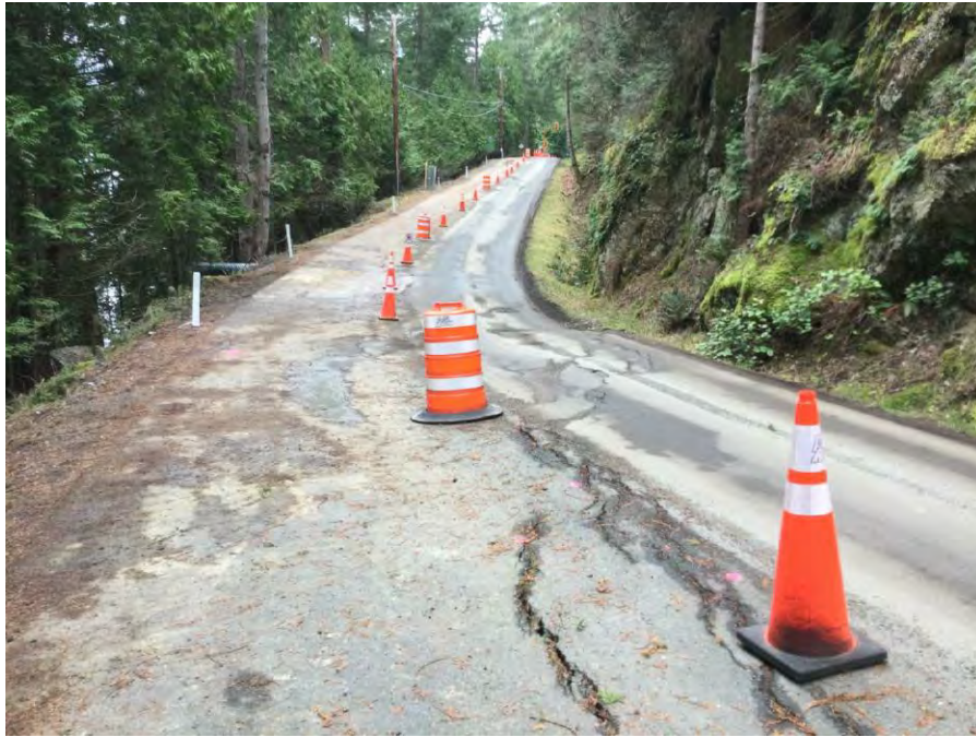
Photo 1 Canal Road - western limit of site with road failure observed. Photo taken looking east on February 17, 2022.
