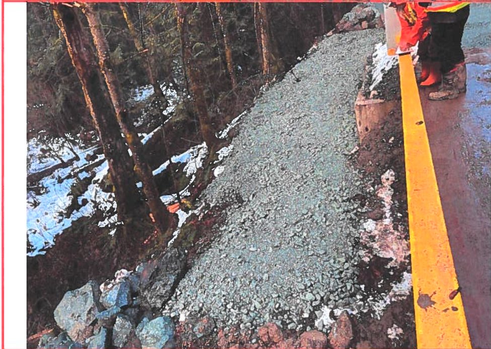
Photo 6: The southwest side of the NW of the bridge. Photo looking northwest.
