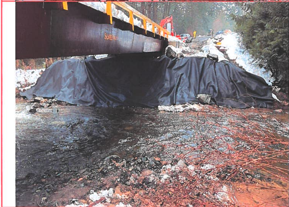
Photo 4: Jan 11, 2022 The entire NW slope was covered by geotextile. Photo looking northwest.
