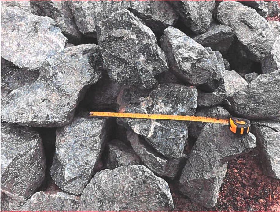
Photo 7: Jan 11, 2022 The small riprap with dimension of about 0.3m (1ft riprap).
