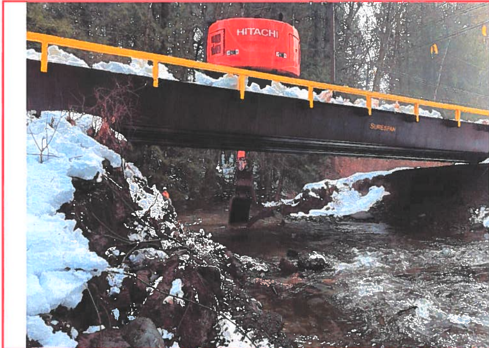
Photo 3: Jan 11, 2022 Observed removal of road failure fragments in process. Photo looking east.
