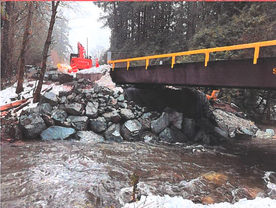
Photo 8: Jan 12, 2022 Upper half of the southwest side of the NW slope was armoured with small ripraps. Photo looking northwest.
