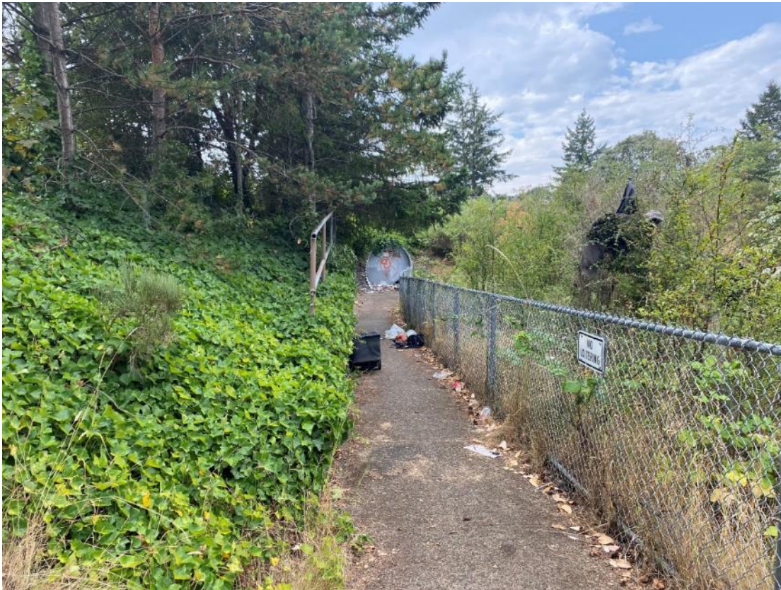
Photograph 3: Pedestrian culvert running underneath Blanshard Street to be filled in that may provide suitable snake denning and/or bat roosting habitat. 10 August 2022.
