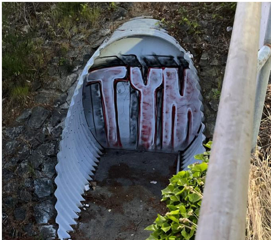
Photo 8: The south side of the culvert to be infilled and the vantage point used by one of the biologists for the bat emergence survey. Photo facing north.
