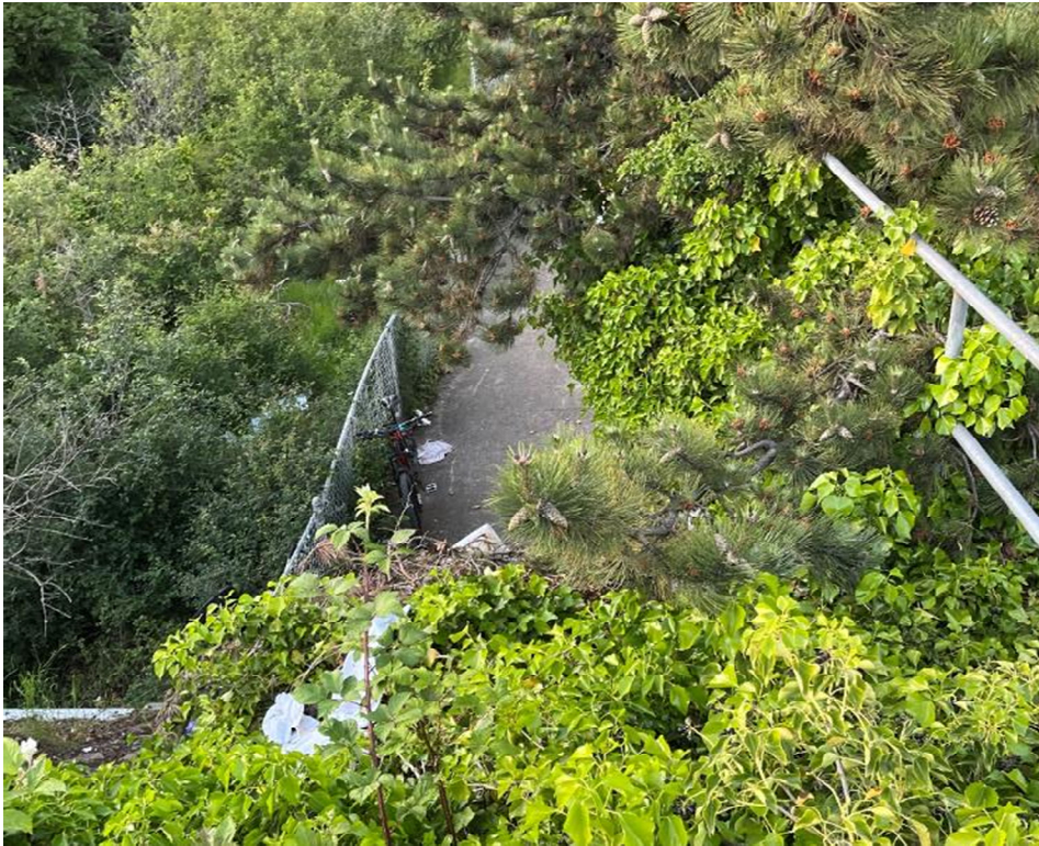
Photo 9: The north side of the culvert to be infilled and the vantage point used by one of the biologists for the bat emergence survey. Photo facing north.
