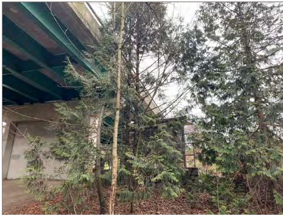
Photo 10: View of western redcedars and bigleaf maples directly south of the north-bound bridge that may need to be removed to accommodate construction.
