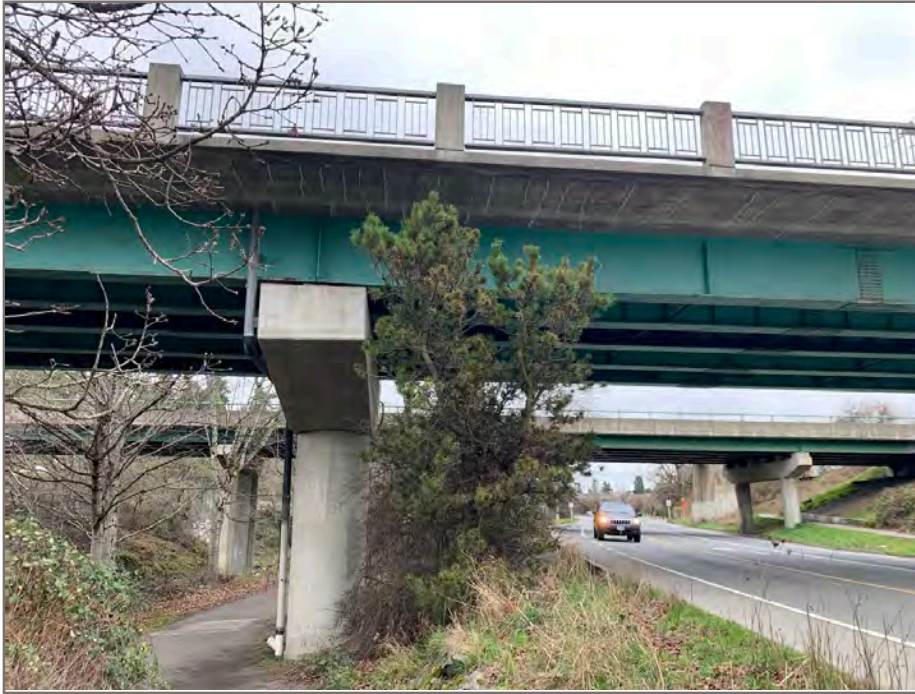
Photo 11: View of shore pine beneath / directly south of the south-bound bridge that may need to be removed to accommodate construction.
