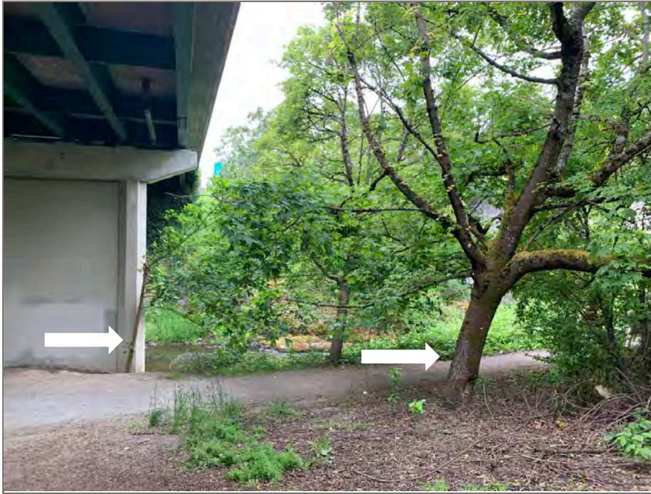
Photo 9: View of bigleaf maple directly adjacent to Bent 3 of the north-bound bridge that may need to be removed to accommodate construction, as well as one other bigleaf maple that may need to be removed to accommodate construction of the rain garden.
