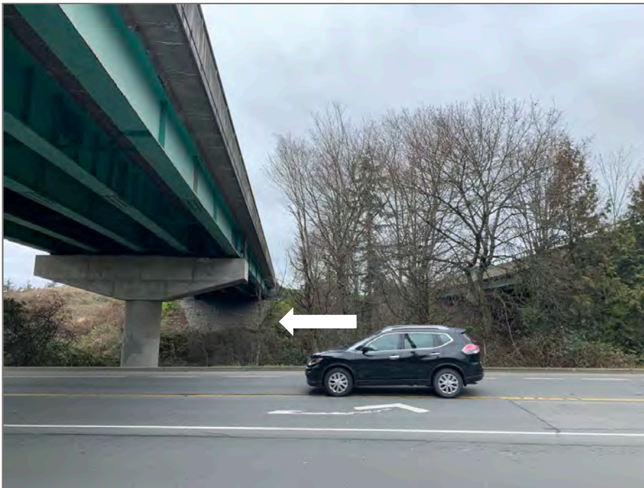
Photo 12: View of bigleaf maple directly north of the south-bound bridge that may need to be removed to accommodate construction.
