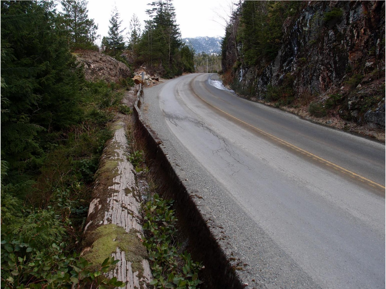
Figure 2: March 2017 Pavement Distress, Looking East
