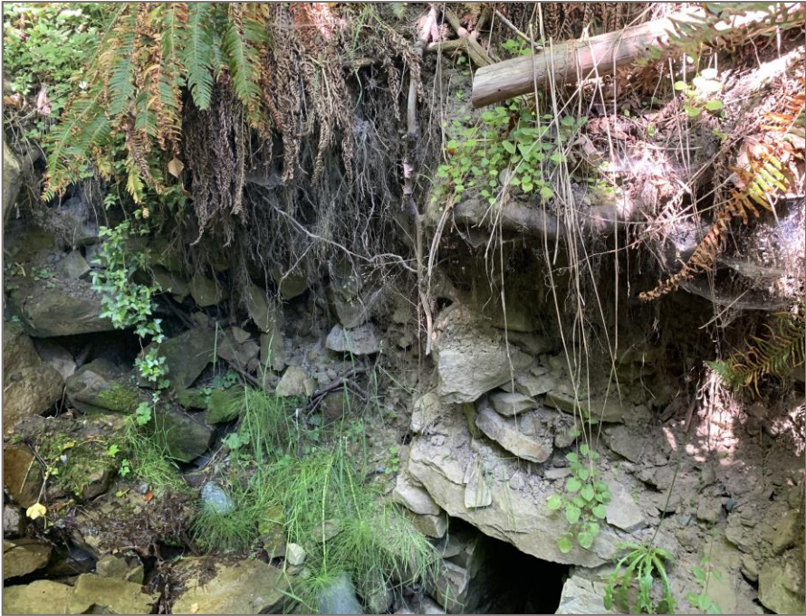
Photo 2: Looking east. View of undercutting (stone cut culvert entry point on west side of culvert/road)
