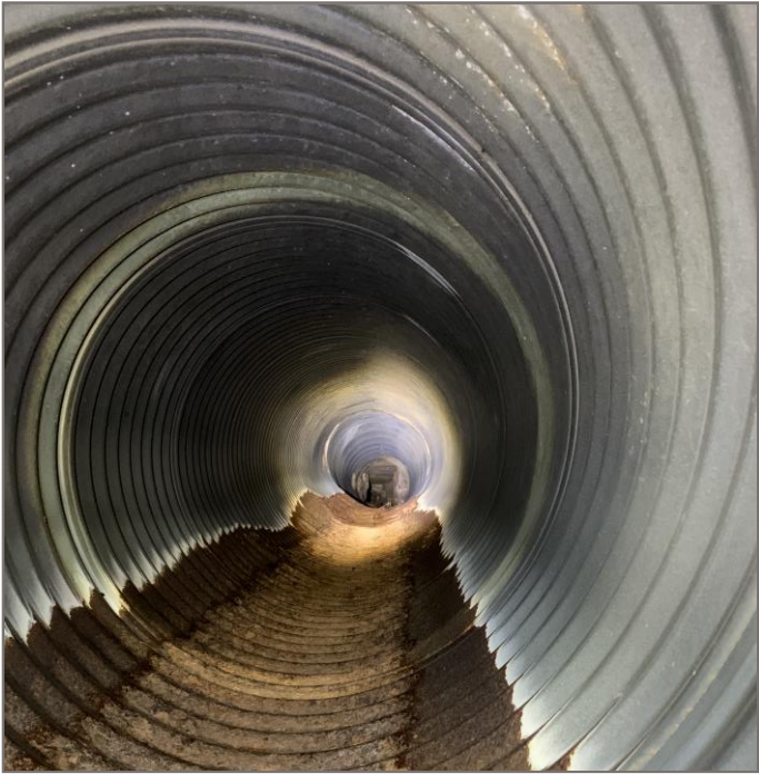
Photo 6: Looking west. View inside round steel pipe culvert showing evidence of deformation
