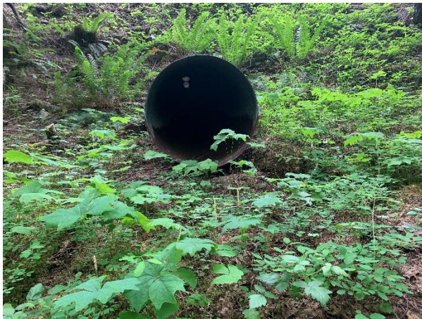
Photo 15: Dry culvert conducting surface drainage under Highway 28, approximately 300 m east of the bridge crossing
