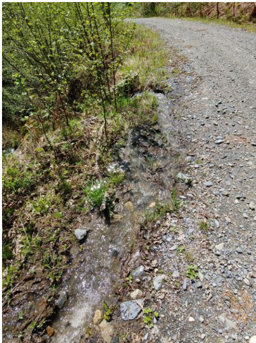
Photo 2-5: Water Flowing South on Road Towards North Crossing Outlet, South View
