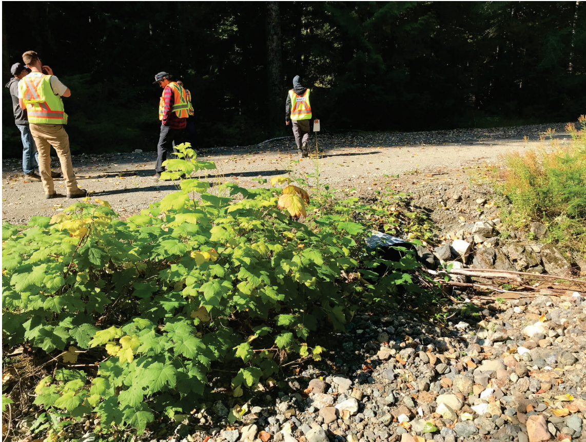
Photo 7: Culvert inlet at km 55.0 partially blocked with gravel, September 21, 2022.
