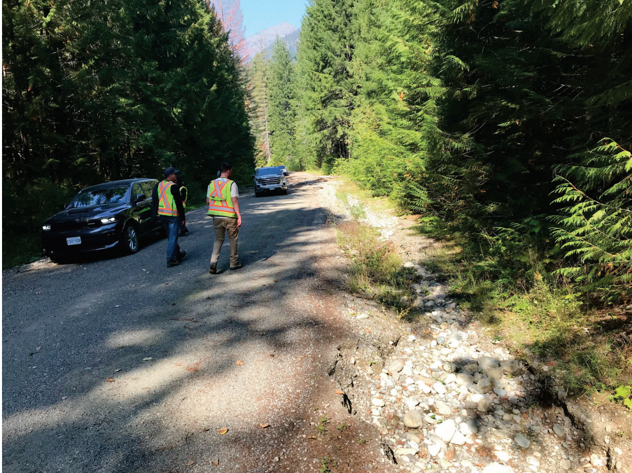
Photo 8: September 21, 2022. Looking north at erosion of the ditch and shoulder on the east side of the road, km 55.0.
