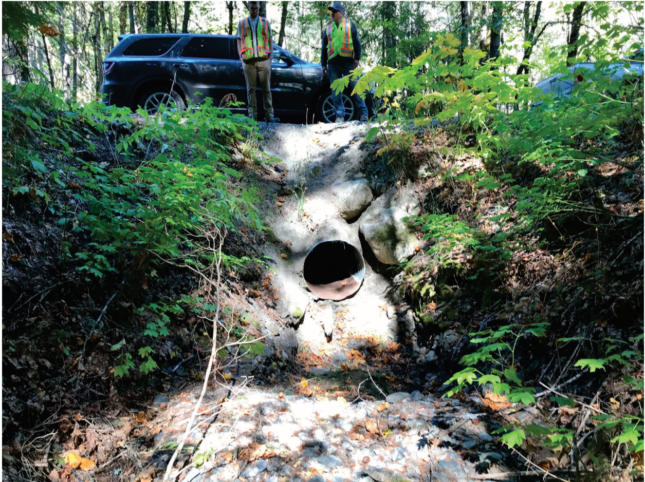
Photo 2: Looking east at the culvert outlet at km 38.4, on September 21, 2022. The culvert inlet was buried.
