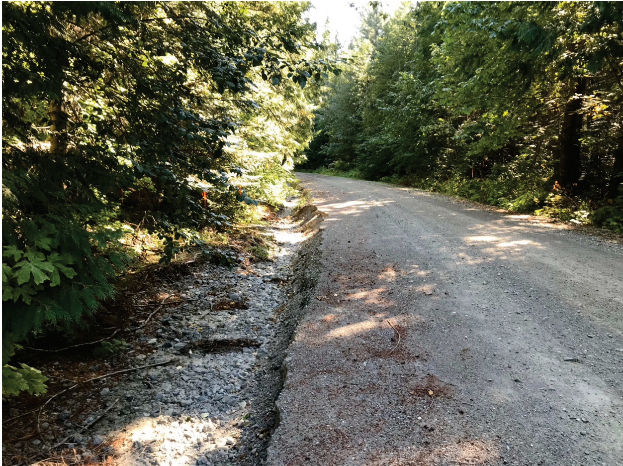
Photo 1: Looking south from km 32.7 of the Silver Skagit Road, on September 21, 2022. Note the erosion damage to the east ditch and shoulder of the road.
