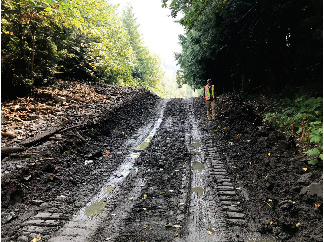
Photo 1: Looking east at the debris fan deposited on the road, Sept 14, 2022.
