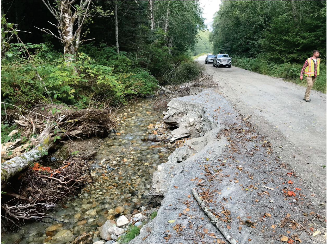
Photo 2: Looking north at the west road edge, km 23.0. Note the erosion of the road edge by the creek.
