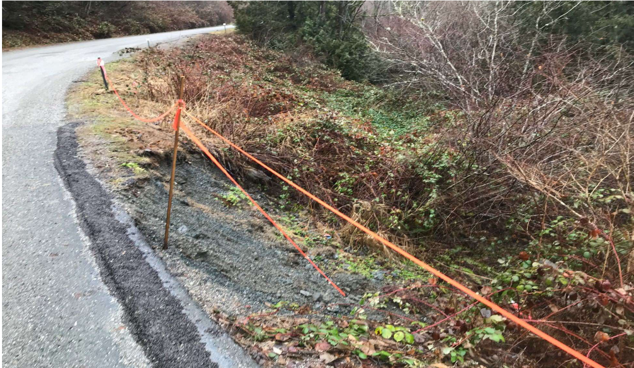
Photo 2: Looking southeast at the area of instability within the subject section
