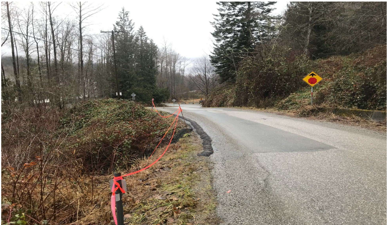
Photo 1: Looking west at the bank repair area (marked with the stakes and ribbon)
