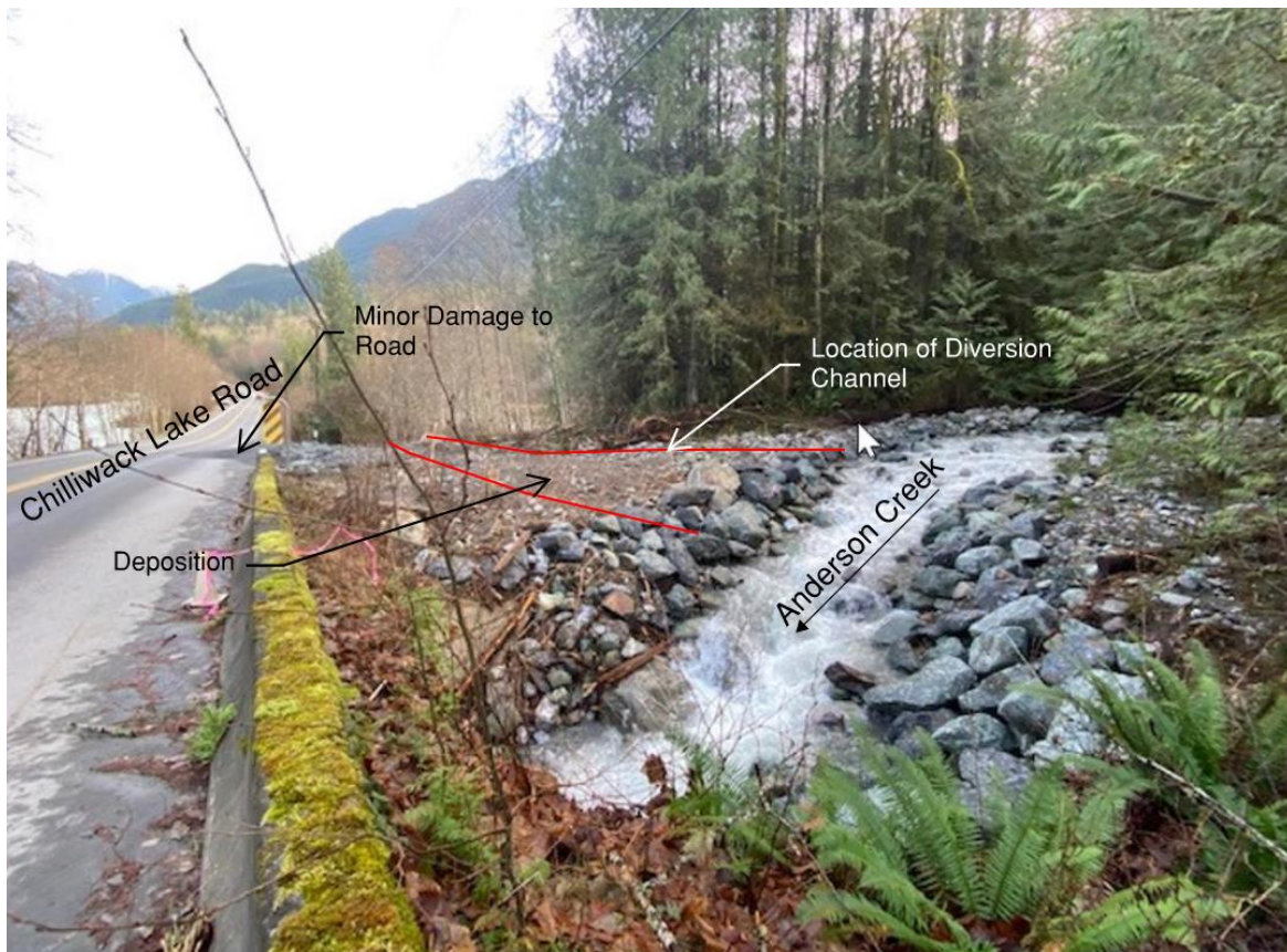
Figure 2. Box Culvert Site after the November 2021 Heavy Precipitation Event
