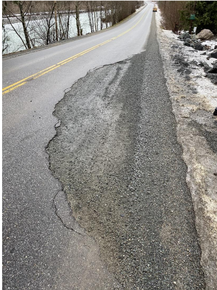
Image 1.1 Asphalt Damage post November 2021 event. Repaired by the Maintenance Contractor.
