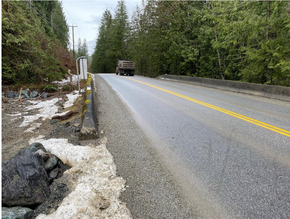
Image 1.2 Temporary Re-Installed Barrie. Non-Compliant to BC MoTI Standards
