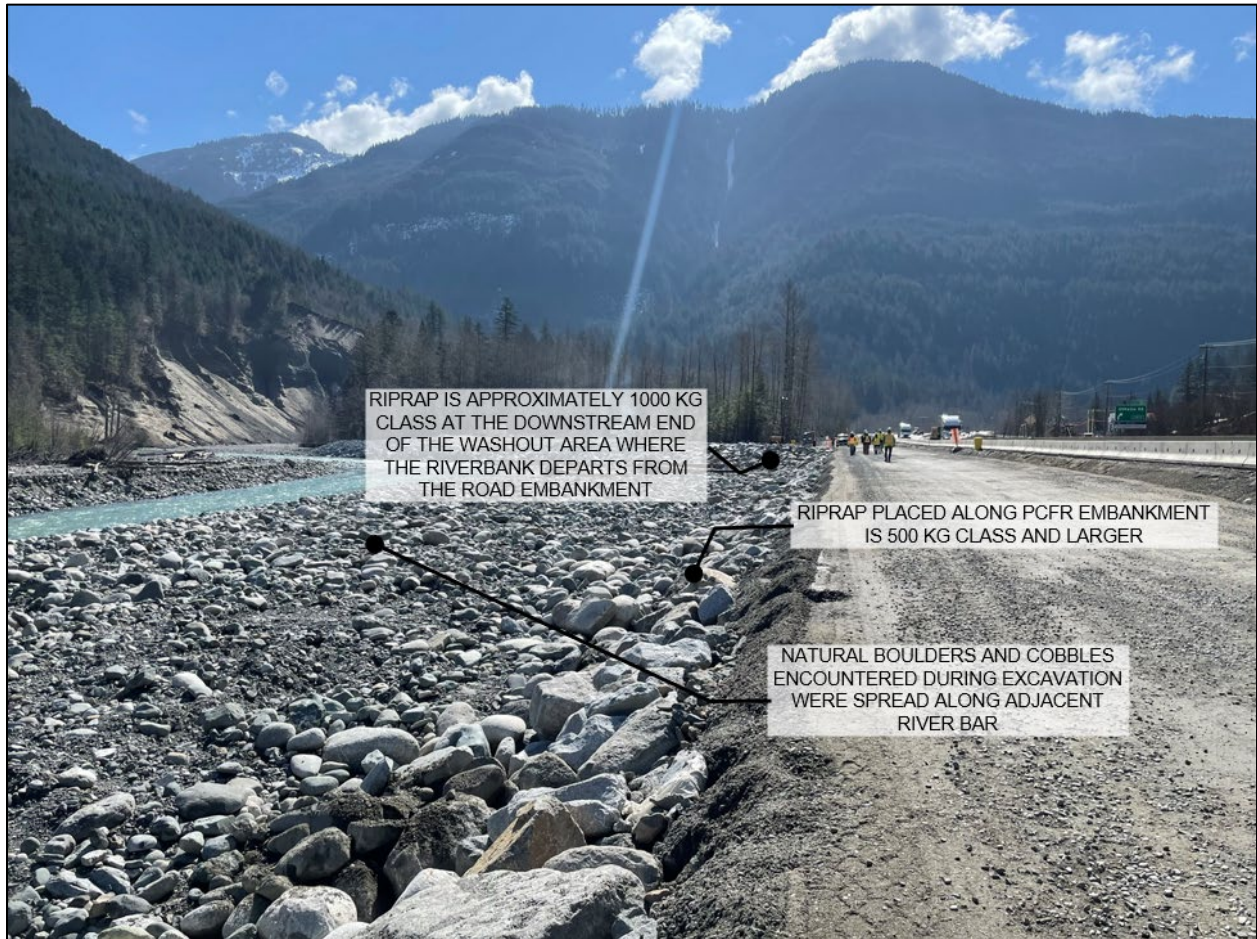
Figure 4-3. View of interim road repairs looking downstream (south). Photo Source: BGC, March 21, 2023.
