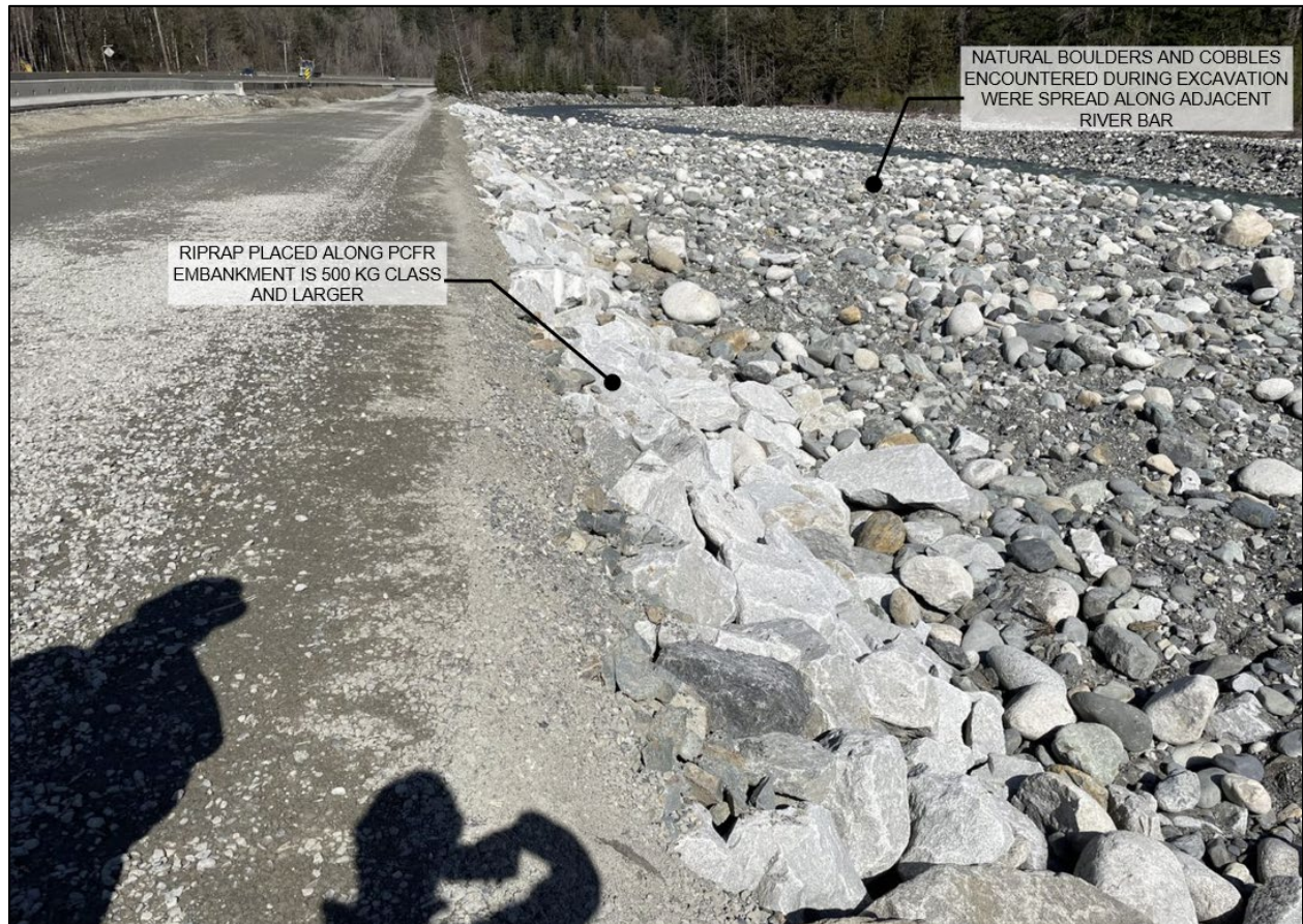
Figure 4-4. View of interim road repairs looking upstream (north). Photo Source: BGC, March 21, 2023.
