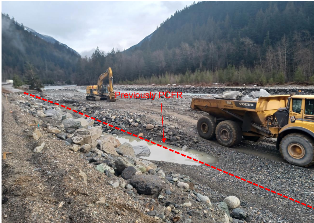
Photograph 3. View looking northeast (upstream) with the red dashed line showing the washout of the PCFR which runs adjacent to eastbound Highway 5 (Photograph provided by MoTI taken on February 27, 2022).
