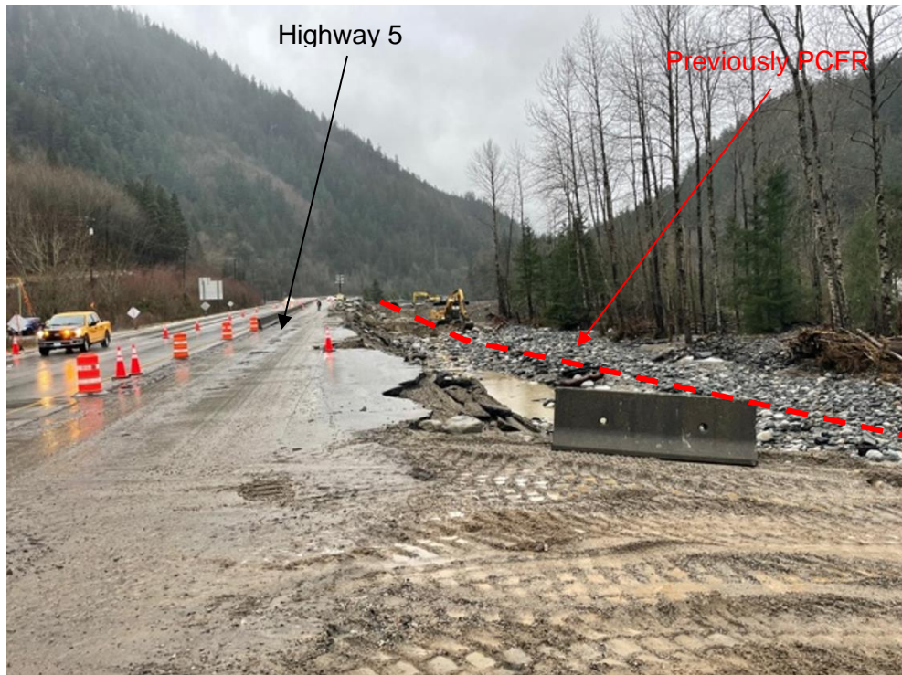
Photograph 6. View looking north (upstream) with the red dashed line showing the washout of the PCFR, which runs adjacent to eastbound Highway 5 (Photograph provided by MoTI taken on March 9, 2022).
