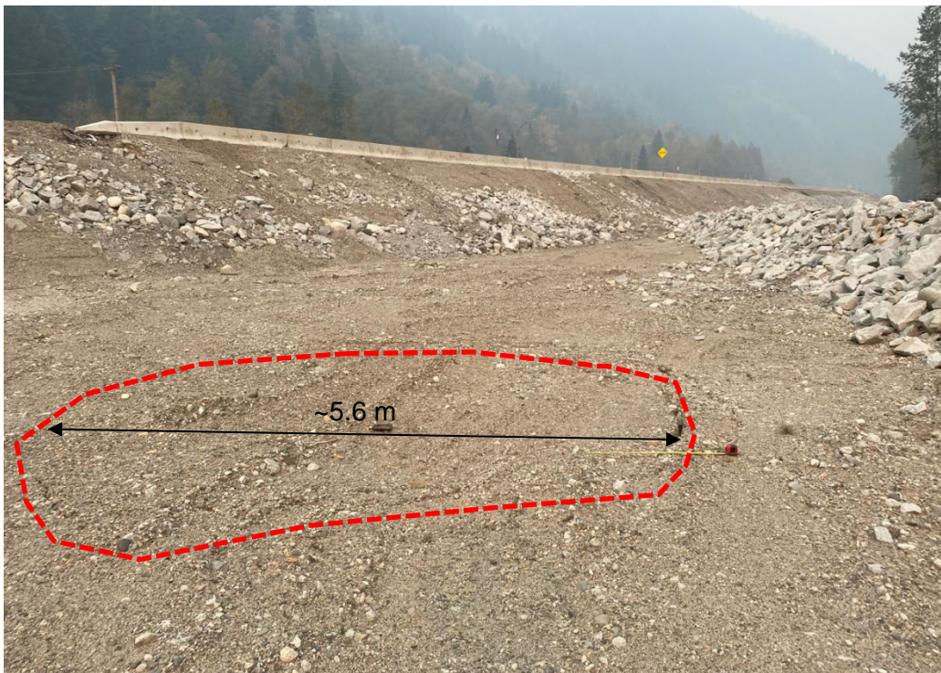
Photograph 16. View looking northwest (upstream) at a localized settlement area (as outlined in red) near the previous PCFR alignment the measuring tape extended to 1 m in the photo (Photograph by BGC taken on October 18, 2022).
