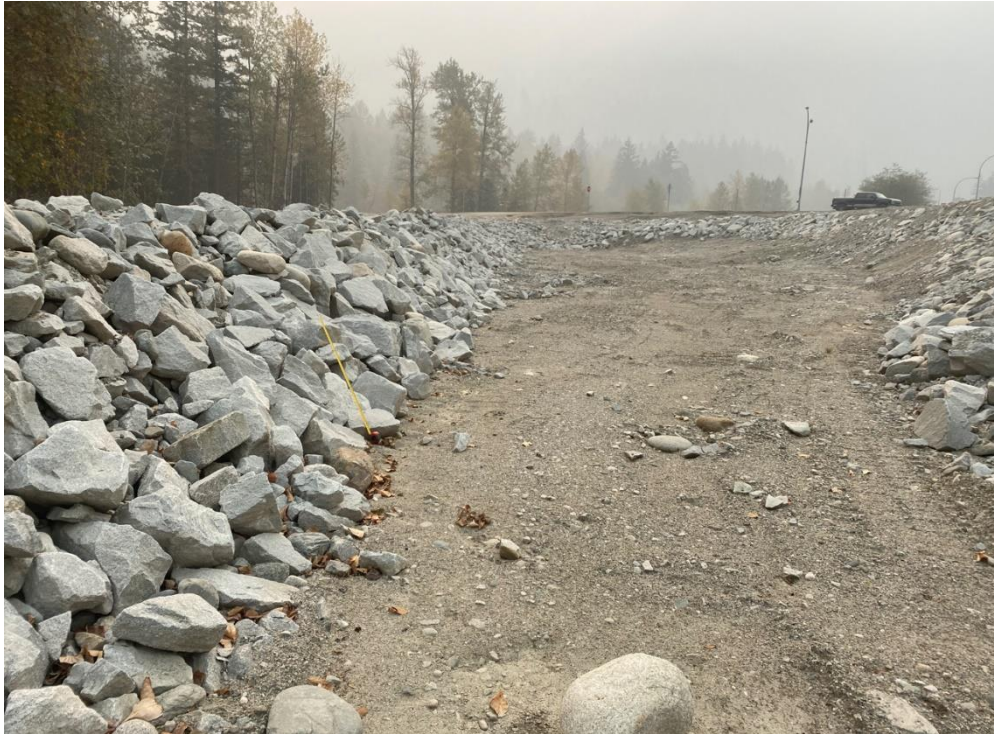
Photograph 15. View looking southeast (downstream) where the previous PCFR alignment with rockfill placed during the response work, the measuring tape extended to 1 m in the photo (Photograph by BGC taken on October 18, 2022).
