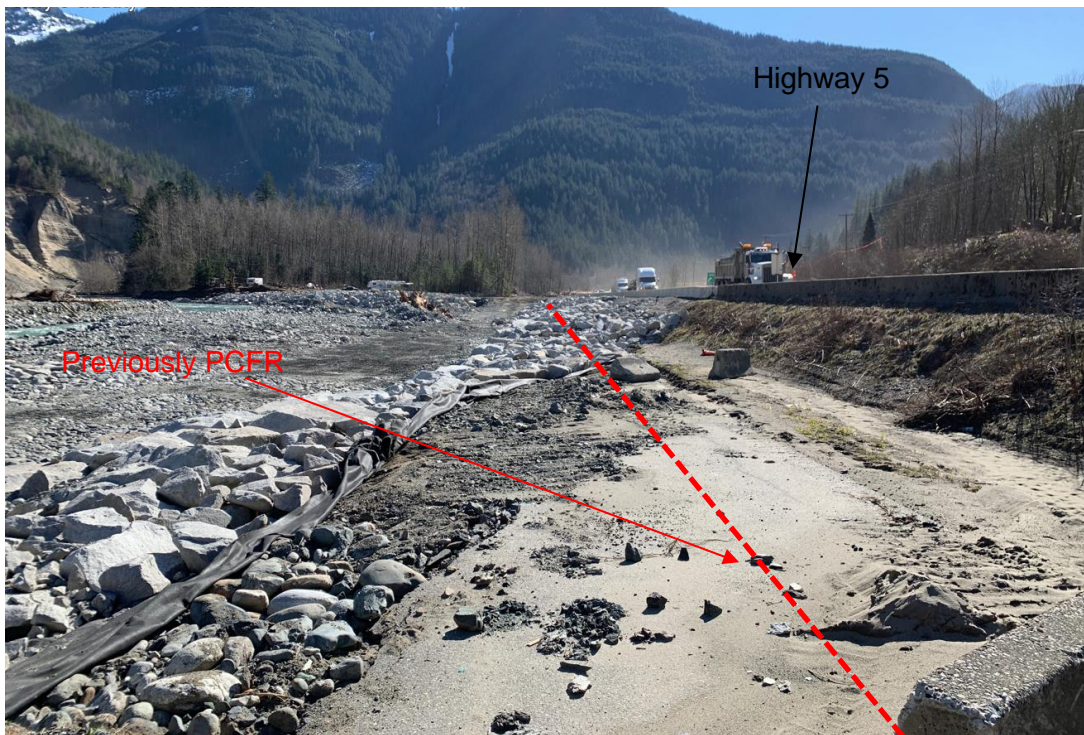
Photograph 4. View looking south (downstream) with the red dashed line showing the washout of the PCFR which runs adjacent to eastbound Highway 5 (Photograph provided by MoTI taken on March 9, 2022).
