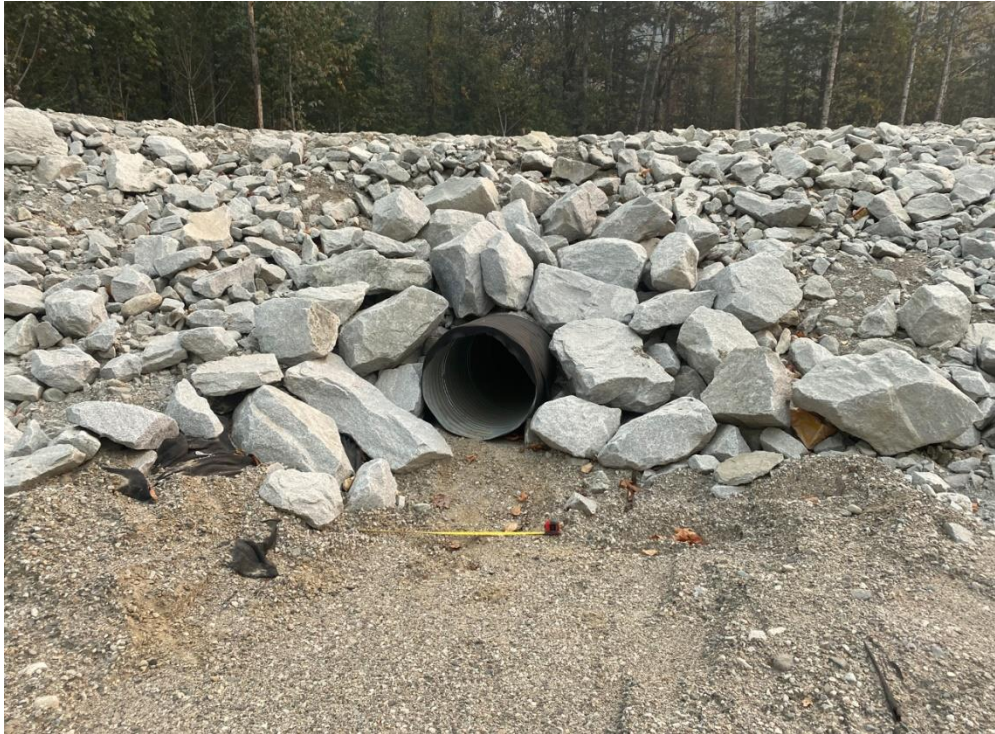
Photograph 17. View looking east at rockfill placed following the initial response work with an 800 mm diameter CSP culvert, the measuring tape extended to 1 m in the photo (Photograph by BGC taken on October 18, 2022).
