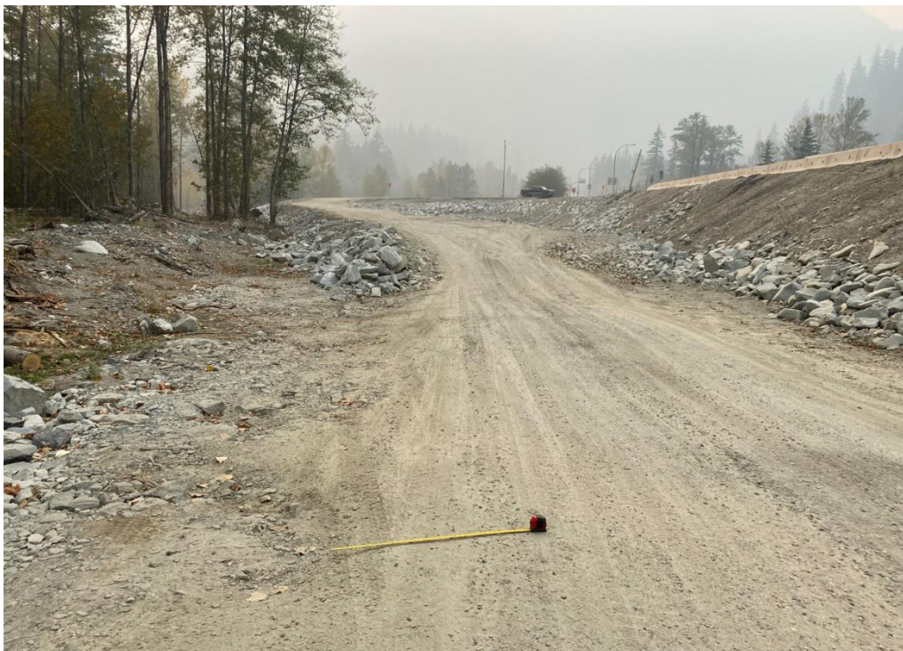
Photograph 14. View looking south (downstream) along the previous PCFR alignment, the measuring tape extended to 1 m in the photo (Photograph by BGC taken on October 18, 2022).
