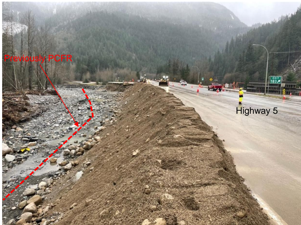
Photograph 2. View looking south (downstream) with the red dashed line showing the washout of PCFR which runs adjacent to eastbound Highway 5 (Photograph provided by MoTI taken on December 11, 2021).
