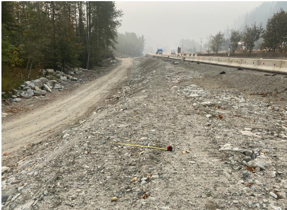
Photograph 10. View looking south (downstream) at embankment fill placed during the initial response work with the measuring tape extended to 1 m in the photo (Photograph by BGC taken on October 18, 2022).
