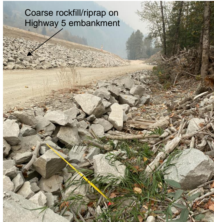
Photograph 13. View looking northwest (upstream) along the previous PCFR alignment the measuring tape extended to 1 m in the photo (Photograph by BGC taken on October 18, 2022).
