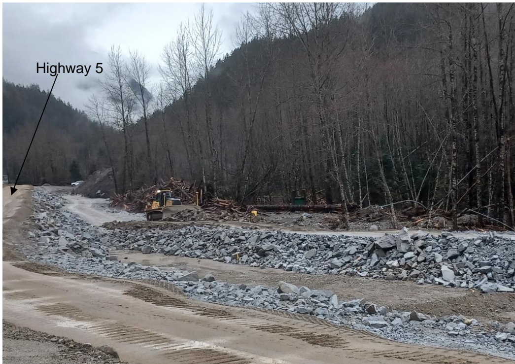
Photograph 5. View looking northeast (upstream) showing rockfill placement along the previous PCFR alignment which runs adjacent to eastbound Highway 5 (Photograph provided by MoTI taken on March 2, 2022).
