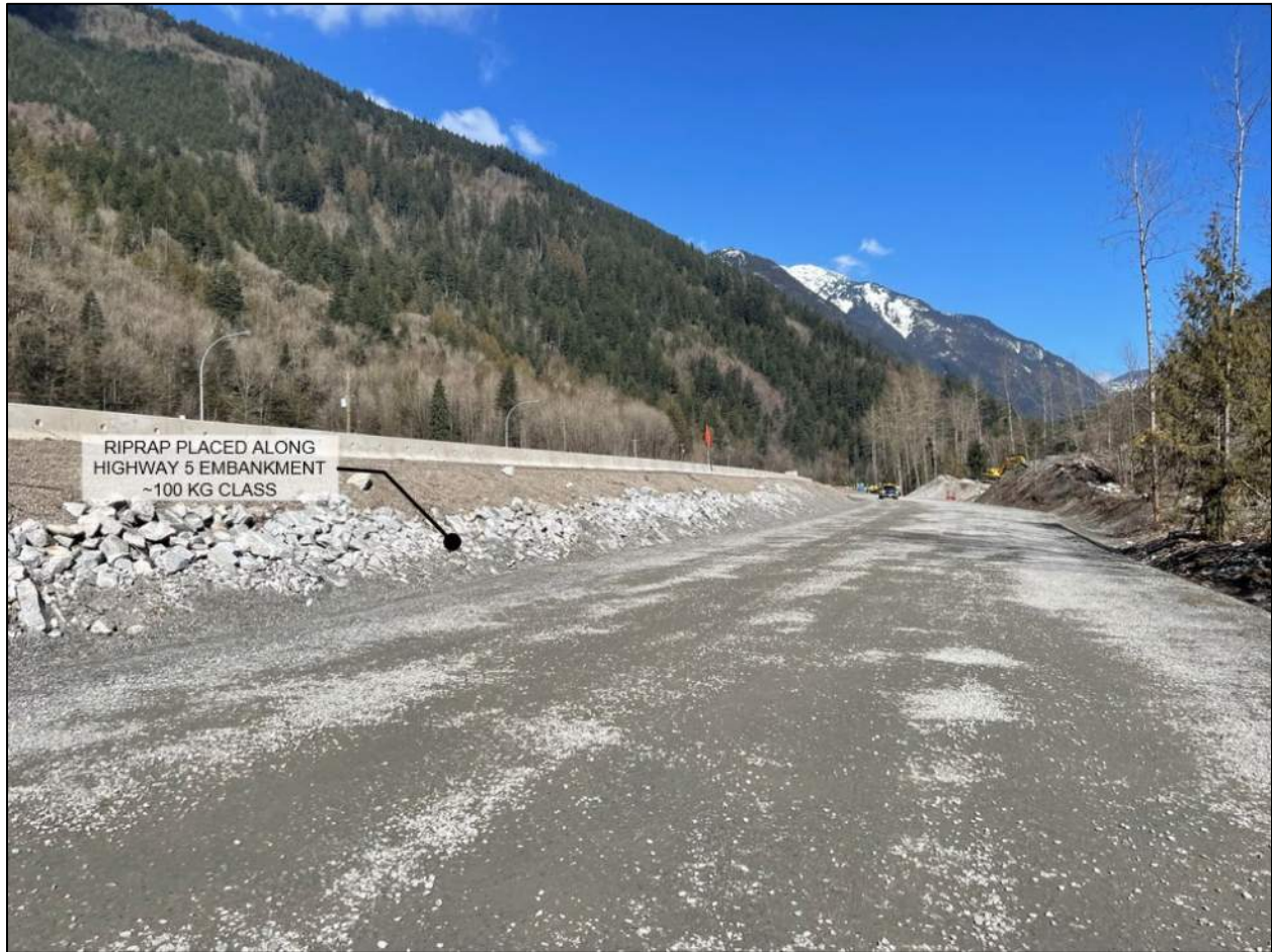
Figure 4-5. View of interim road repairs looking north near the Othello interchange. Photo Source: BGC, March 21, 2023.
