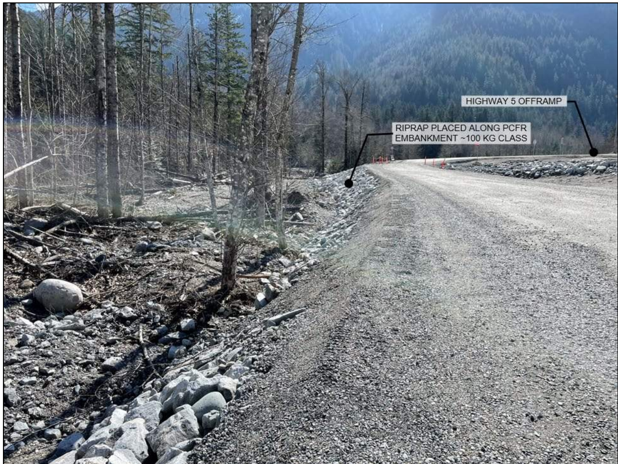
Figure 4-6. View of interim road repairs looking south near the Othello interchange. Photo Source: BGC, March 21, 2023.
