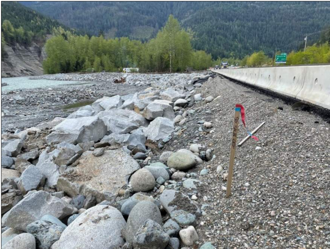
Figure 4-1. Looking downstream along emergency bank protection place on the right bank of the Coquihalla River. Photo Source: BGC, May 9, 2022
