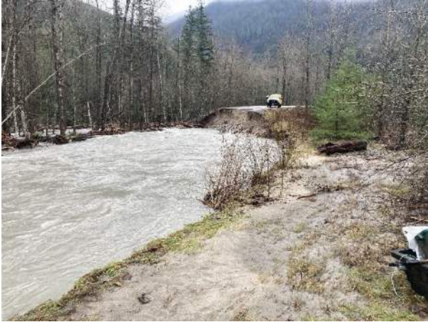
Photo 1. Looking south towards Peers Creek Road washout along Coquihalla River in November 2021.
