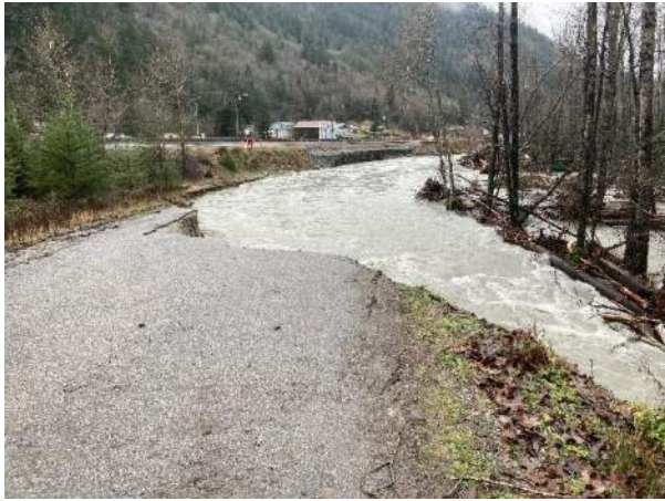
Photo 2. Looking north from Peers Creek Road washout along Coquihalla River in November 2021.
