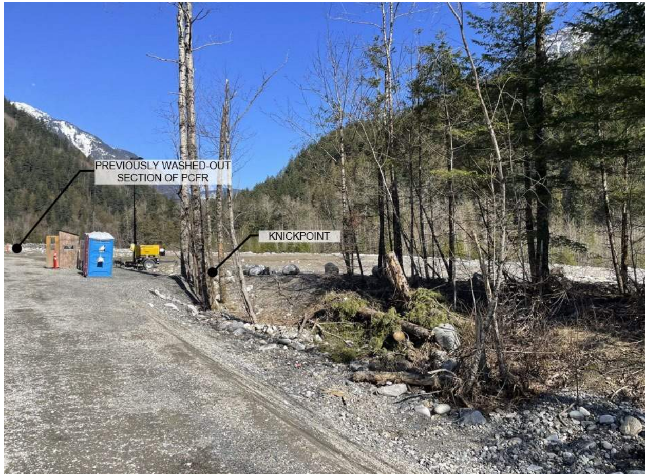
Figure 5-2. View of potential knickpoint immediately south of previously washed-out section of PCFR. Photo Source: BGC, March 21, 2023.
