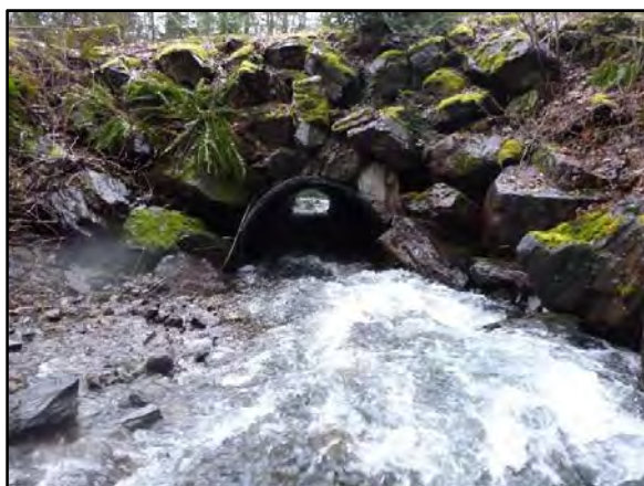
High flow velocity observed at the Rockwell Drive culvert inlet.
