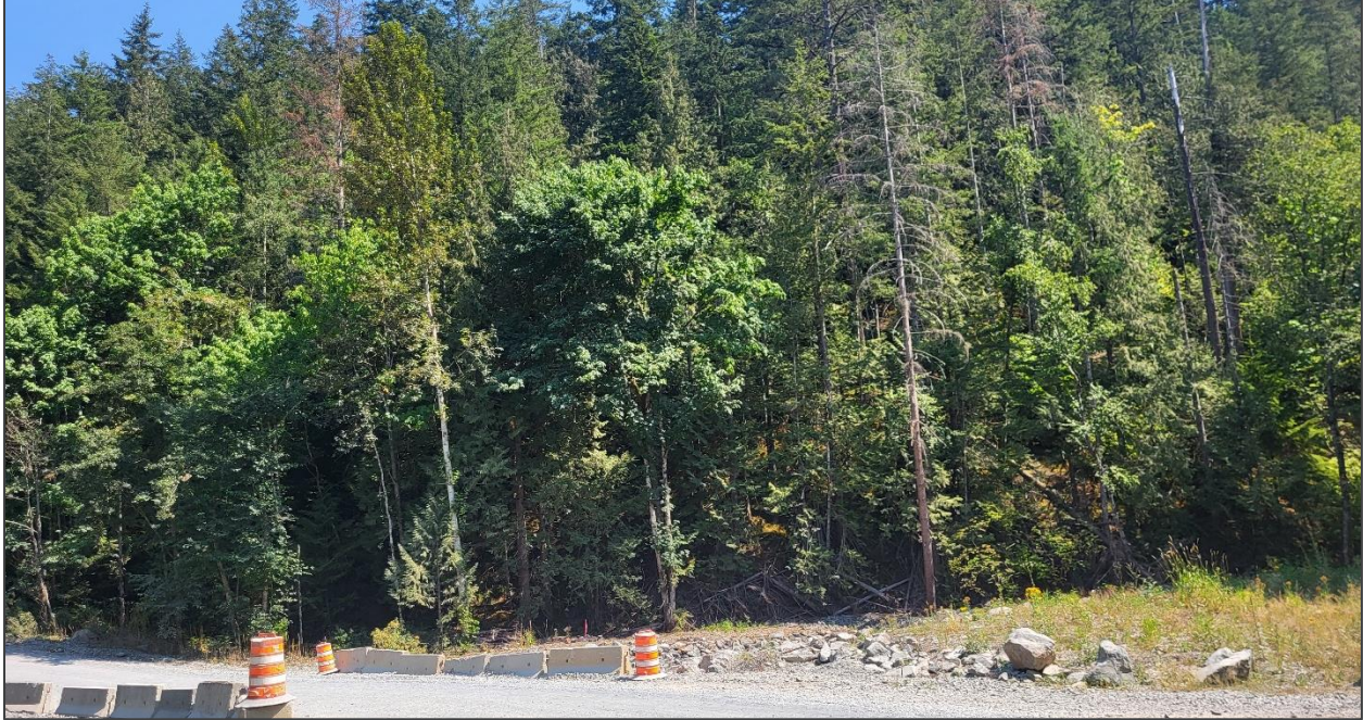
Figure 2. DF#4 - sample image of the soil erosion and steep terrain above the Hick's Lake Road (view from the West to the East).
