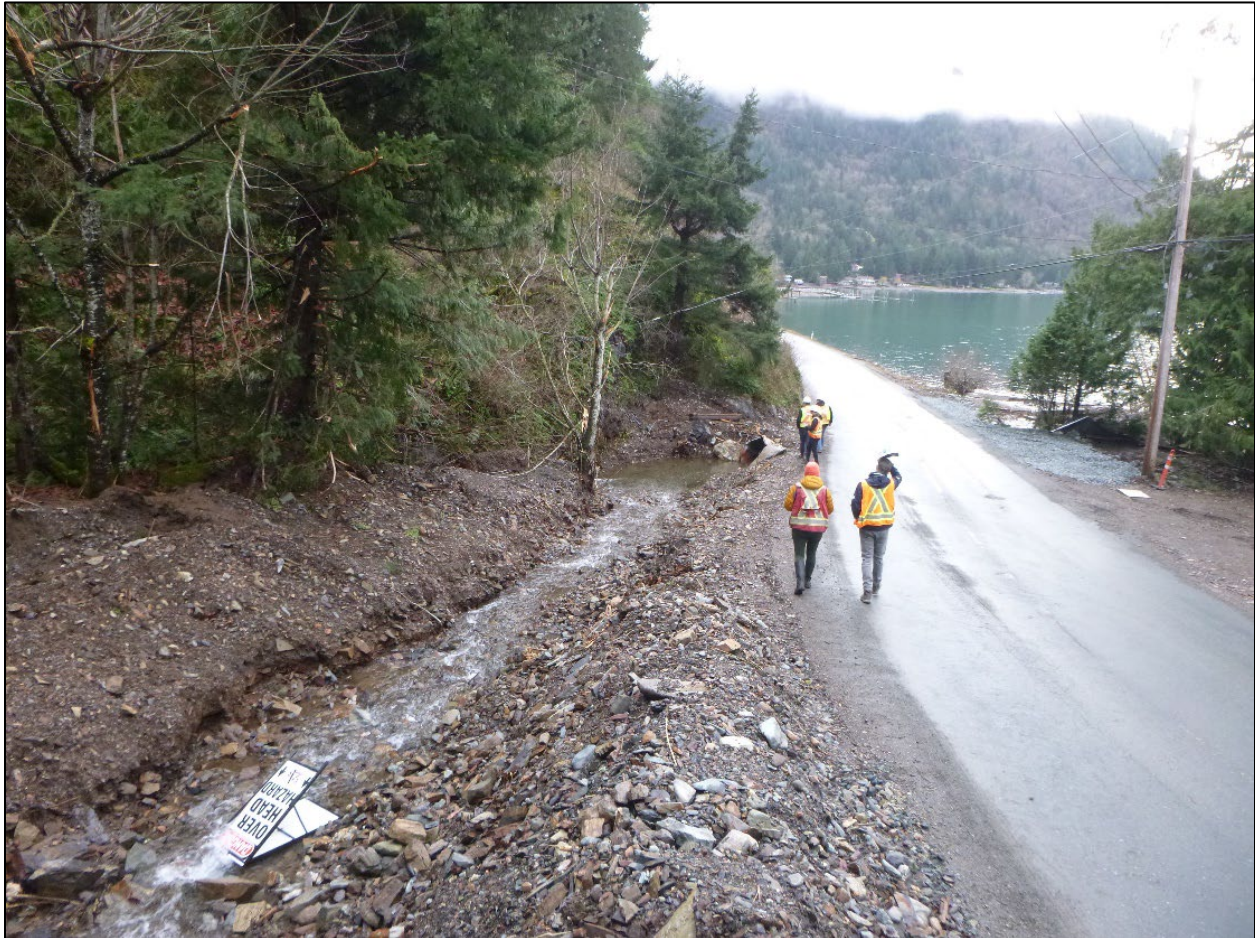
Figure 2 Downstream view of site DF2 showing erosion and debris along Rockwell Drive (December 14, 2021).
