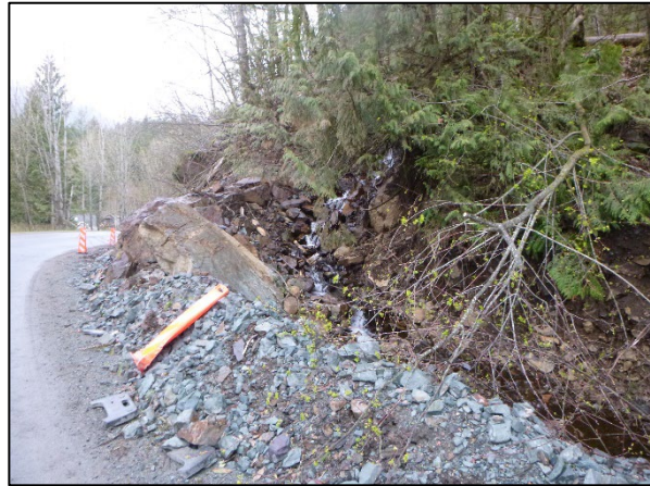
Photo 2: Creek avulsion directed back to the south via a berm along Rockwell Drive.
