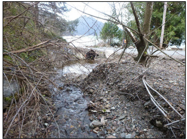
Photo 4: Downstream view of the Rockwell Drive culvert inlet where the roadside ditch and altered channel converge.
