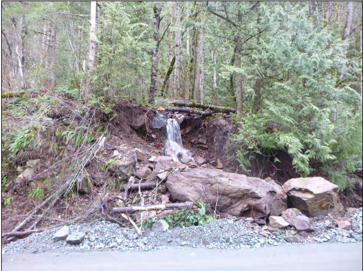
Figure 3 Watercourse avulsion at site DF3 (December 14, 2021).
