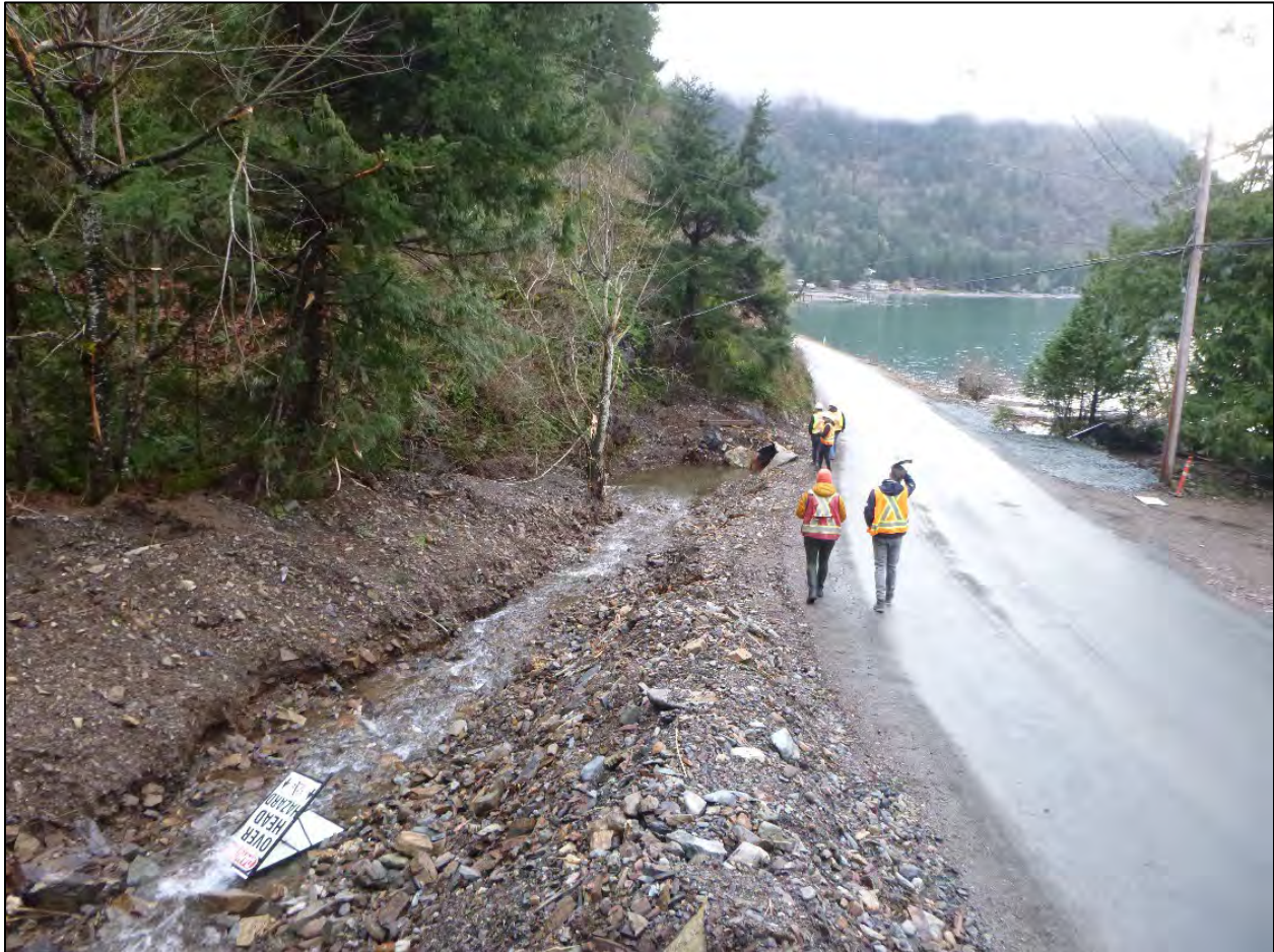
Figure 2 Downstream view of site DF2 showing erosion and debris along Rockwell Drive (December 14, 2021).
