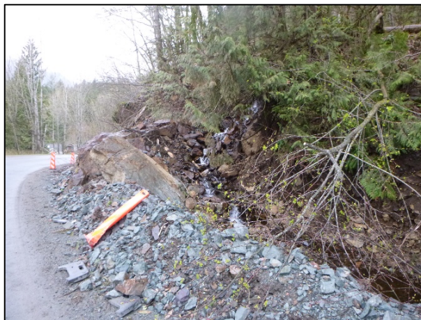
Creek avulsion directed back to the south via a berm along Rockwell Drive.
