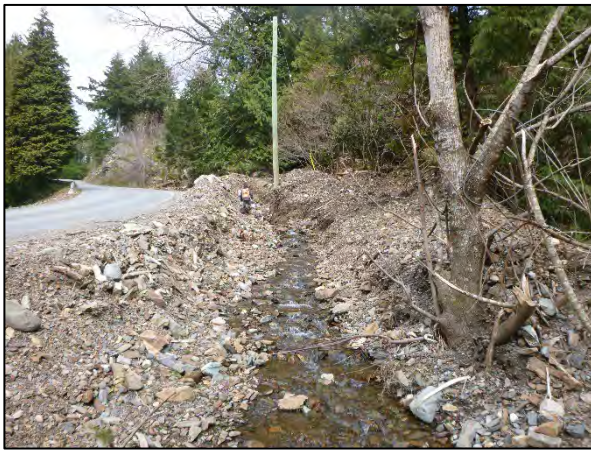
Photo 3: Upstream view of the roadside ditch along Rockwell Drive upstream of the culvert.
