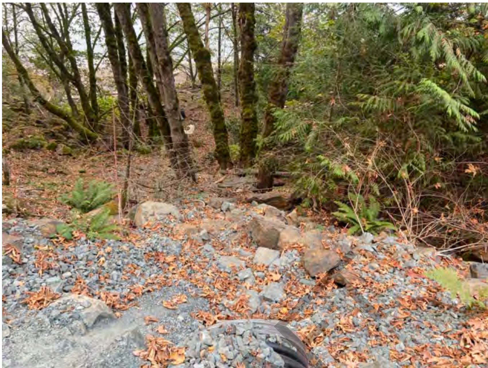
Photo 7 DF3-View west-southwest of culvert outlet and steep terrain descending to Harrison Lake on the west side of Rockwell Drive
