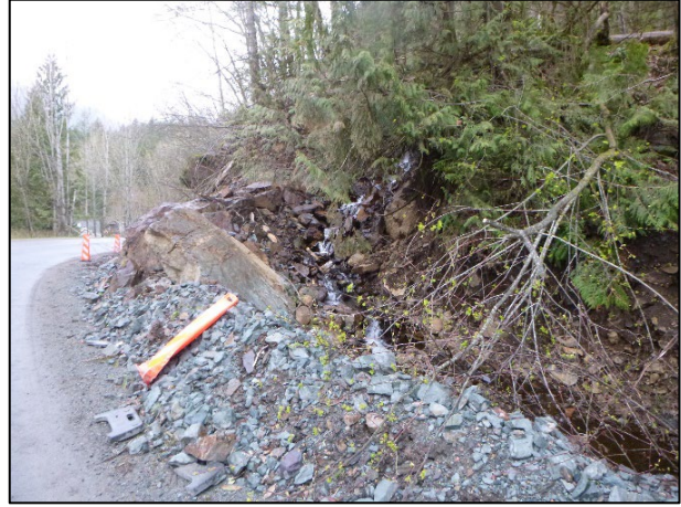
Creek avulsion directed back to the south via a berm along Rockwell Drive.
