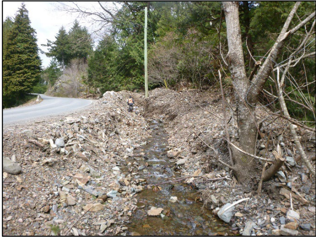
Upstream view of the roadside ditch along Rockwell Drive upstream of the culvert.
