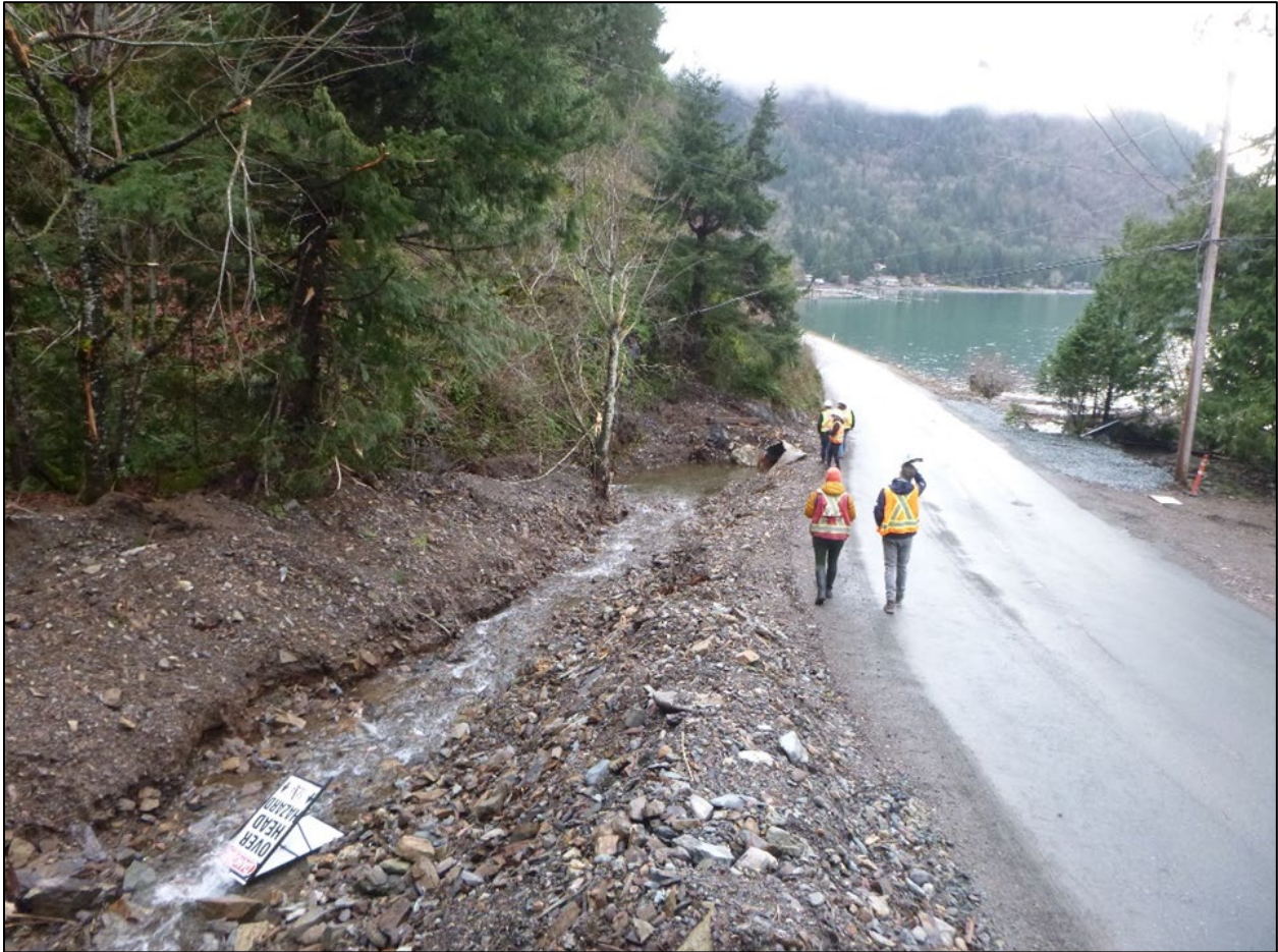
Figure 3 Downstream view of site DF2 showing erosion and debris along Rockwell Drive (December 14, 2021).
