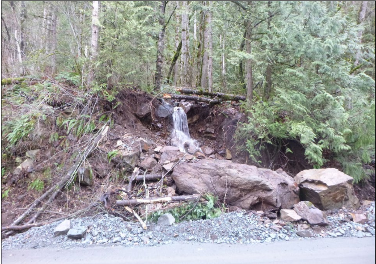
Figure 4 Watercourse avulsion at Site DF3 (December 14, 2021).
