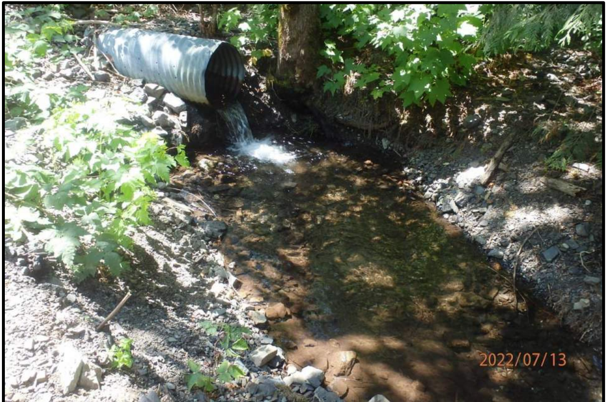
Figure 3. Culvert outlet is elevated at Teapot Hill east culvert.
