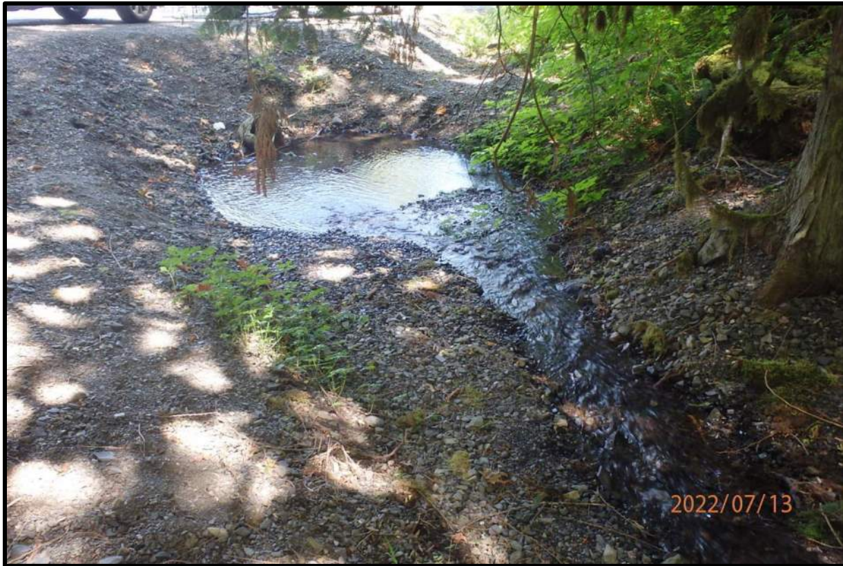
Figure 4. Low-gradient stream channel at the inlet to Teapot Hill east culvert, upstream of Columbia Valley Road.
